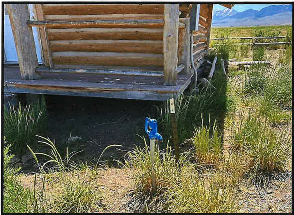
Photo 2- Facing north frost free spigot in foreground. There were two spigots at the cabin neither one was operational at the time of the field examination.
