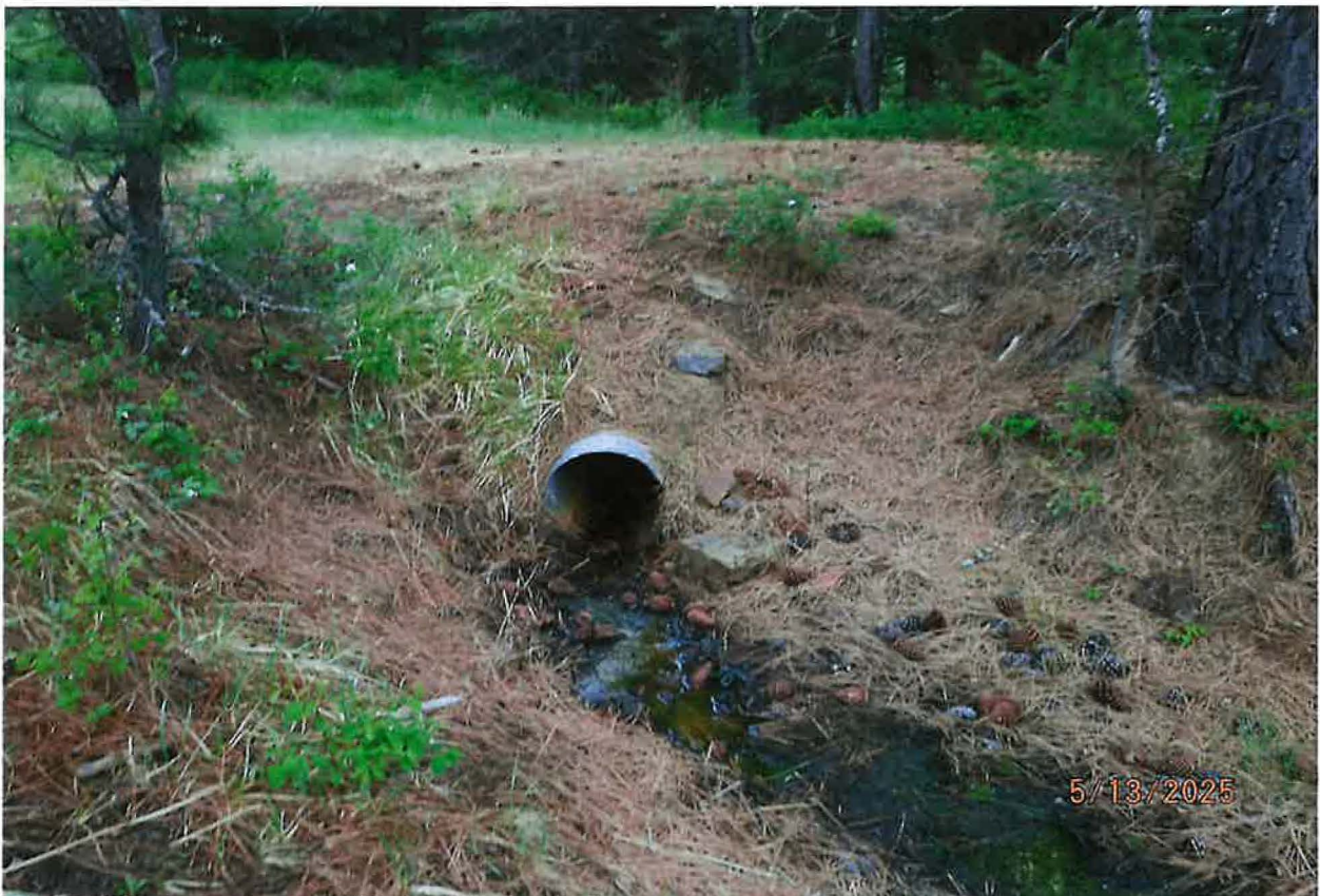
STORAGE POND OVERFLOW DEVICE – METAL CULVERT BENEATH ROAD ALLOWS OVERFLOW WATER TO CONTINUE DOWNSTREAM IN BASIN
