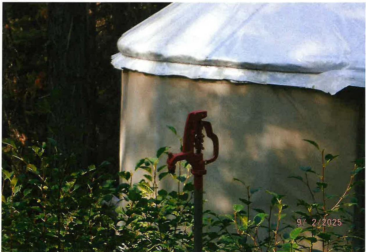
DOMESTIC POU – HYDRANT SET AT 8 FT ELEVATION FROM GROUND – WINTERTIME USE WITH SNOW LEVEL RESULTS IN HYDRANT AT 2 FT ABOVE SNOWPACK
