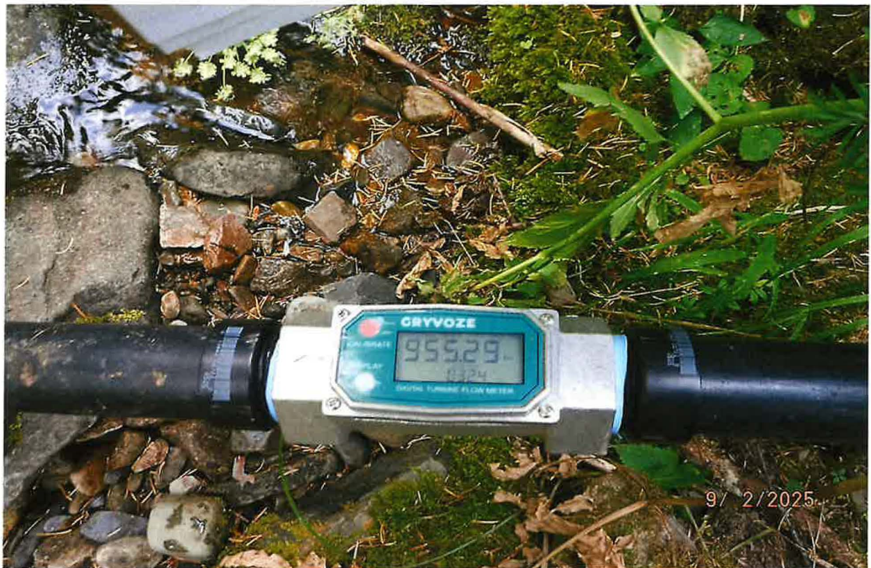
POWER SYSTEM – ELECTRONIC FUEL METER INSTALLED INLINE AT OVERFLOW DISCHARGE FROM POWER UNIT – 32.4 GPM OBSERVED AT TIME OF EXAM WITH TOTAL GALLONS REGISTERING FOR TOTAL RUNTIME GALLONS ON DAY OF EXAM
