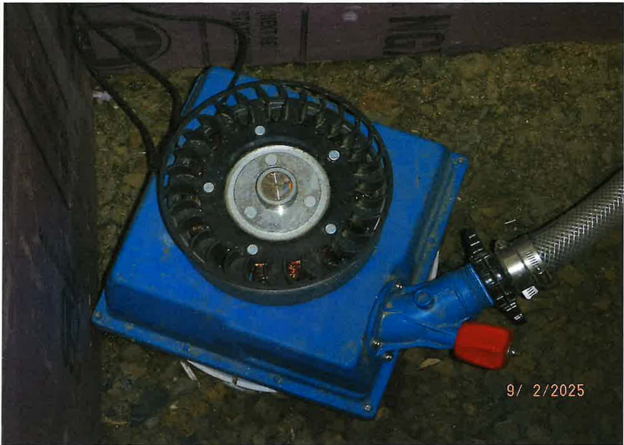
POWER POU – TURGO WHEEL MICRO-HYDRO UNIT; 1 SPHERE VALVE ADJUSTABLE NOZZLE CREATES 30-50 Wh DEPENDENT ON SETTING
