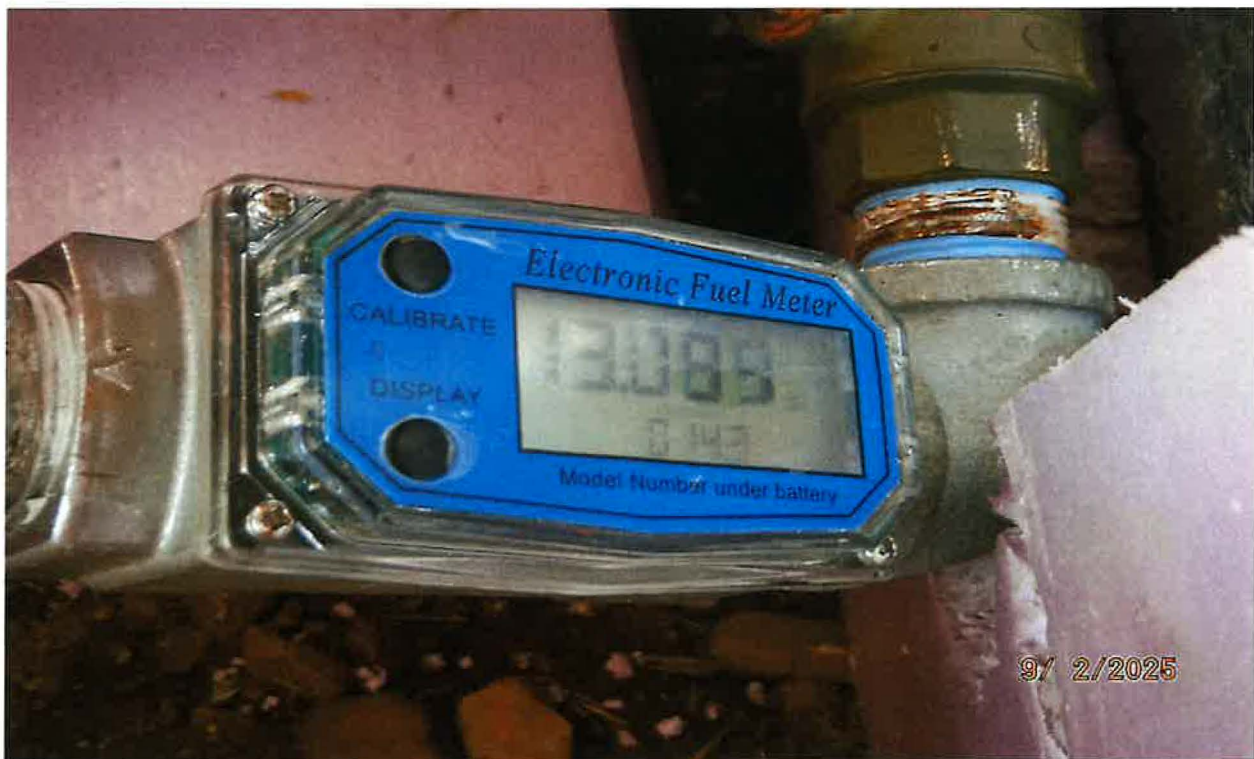
DOMESTIC POU – LARGE YURT (END OF 200-FT + 700-FT 1-INCH POLY) OVERFLOW DISCHARGE PIPE WITH ELECTRONIC FUEL METER FLOWMETER INSTALLED. OBSERVED 14.3 GPM FROM LARGE YURT FLOW RESULTING FROM GRAVITY FLOW SYSTEM THAT ROUTES VIA SIDE-HILL FROM STREAM TO LARGE YURT
