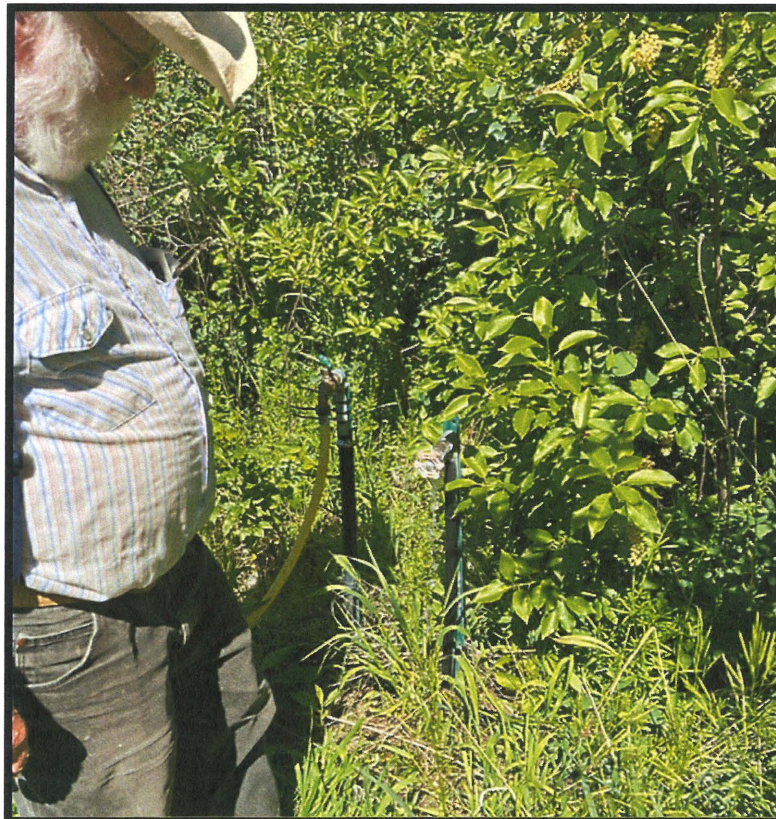
Photo 5- Facing north at the western spigot in the SWNW of Section 20. Only the right spigot is connected to the spring source the spigot on the left is connected to the system for 74-16241, for domestic irrigation use.
