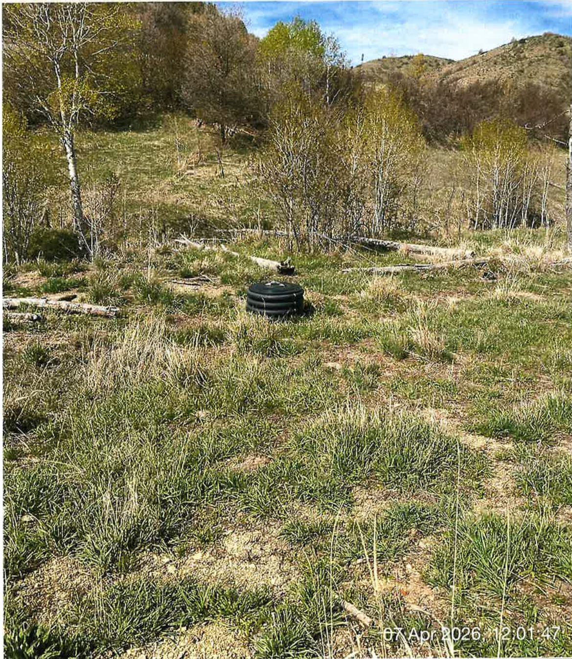
Point of diversion. Water is conveyed by gravity through buried pipe to the stockwater trough just down the hill. (GPS coordinates on photo have error, exact location is correct on the map)
