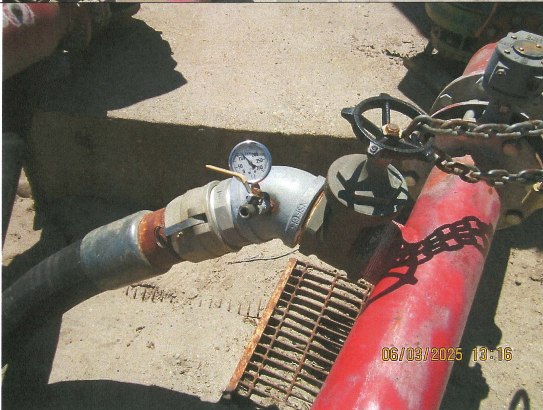
Figure 16. Pressure gage on pipe going to Hill Road and lockable controllable valve.
