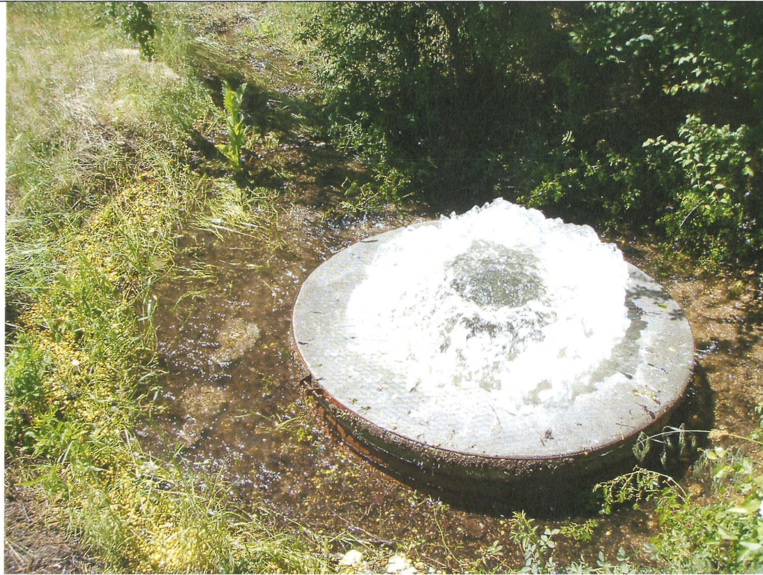
Figure 5. Bubbler screens trash before entry into mainline.
