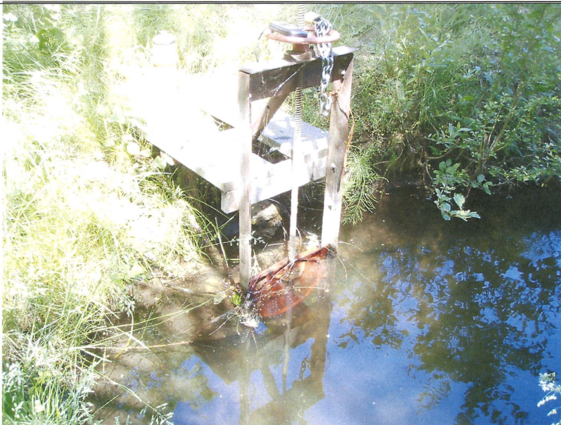
Figure 2. A lockable controllable Waterman headgate at the diversion point from Porter Creek leads to the measurement weir and pipeline headworks.
