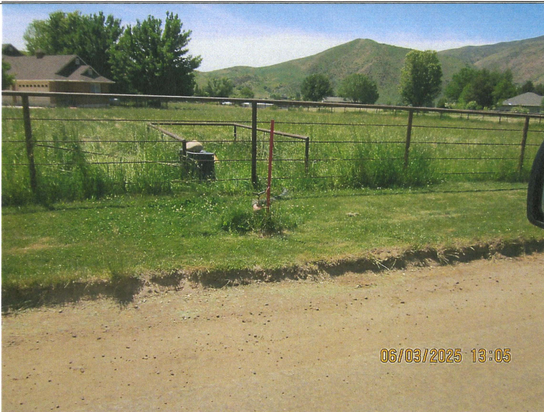
Figure 10. Stubb valve to 48 Hill Creek Road.
