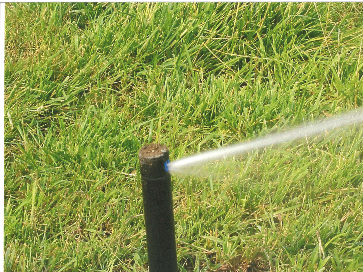
Figure 5. Pasture irrigation consists of Hunter rotors equipped with blue 5 gpm nozzles designed for 30 gpm per zone with 6 sprinklers per zone.
