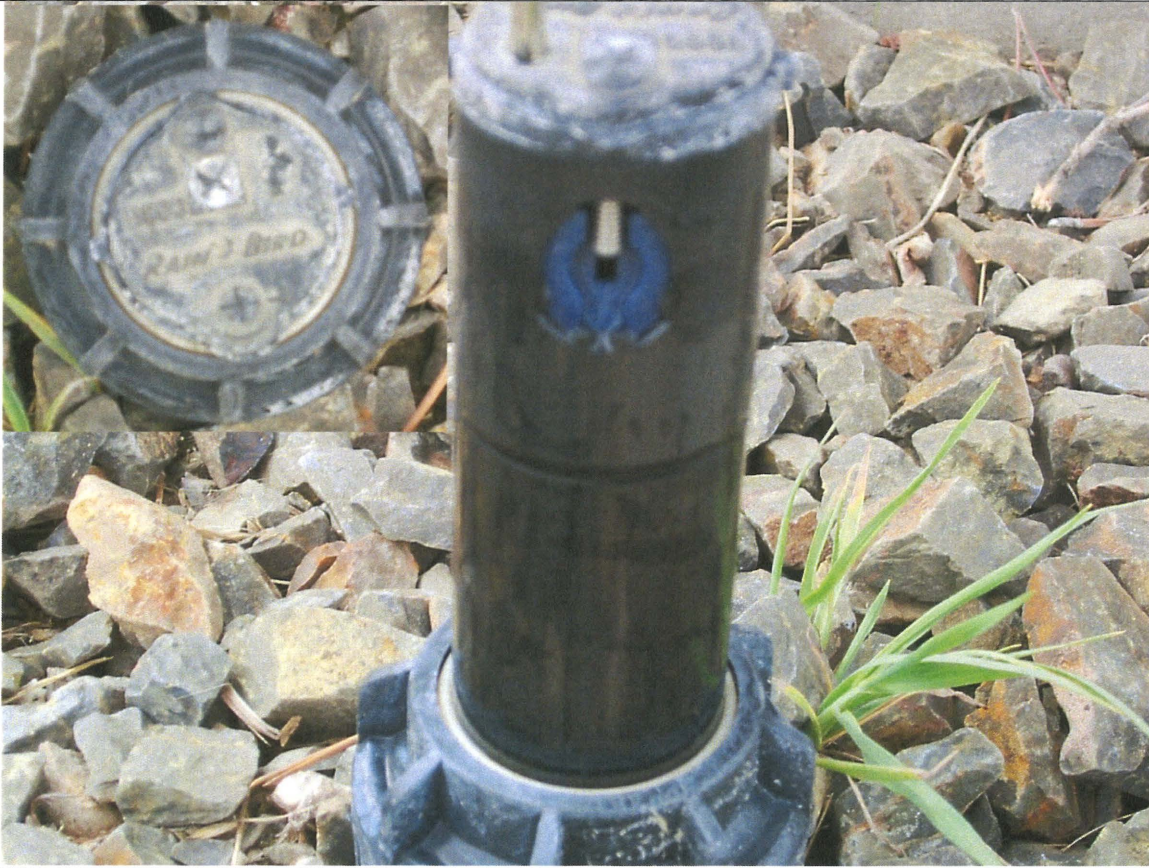
Figure 4. Lawn irrigation consists of Rainbird 5000 rotors. There are 10 zones of sprinklers and 3 zones of dripline. The largest zone consisted of 9 sprinklers.
