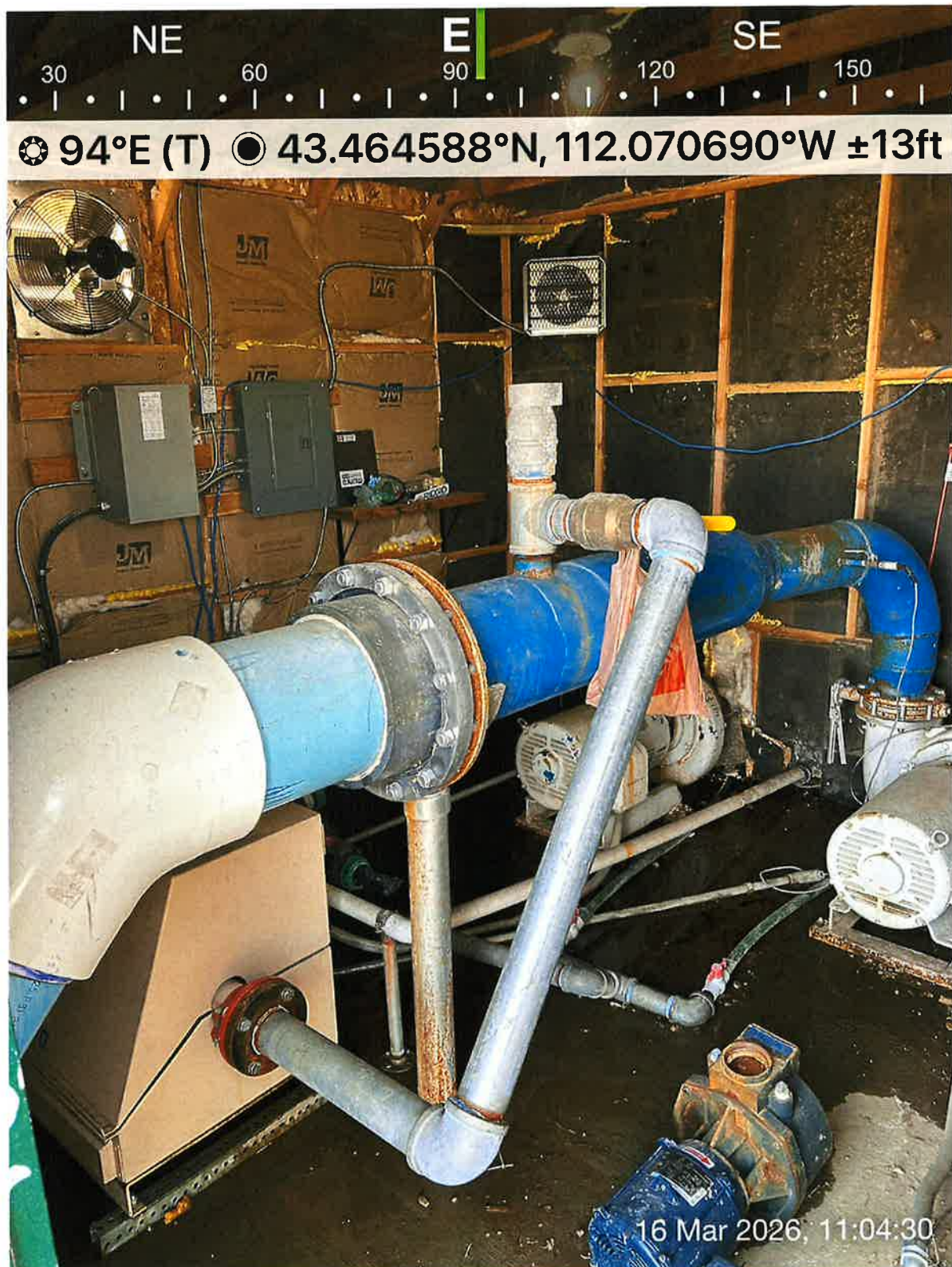
Picture of the inside of the pump house. Two electric motors divert water into a single mainline
