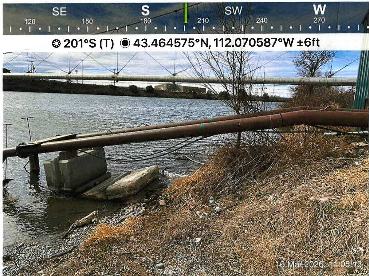
Pump intake from the Snake River
