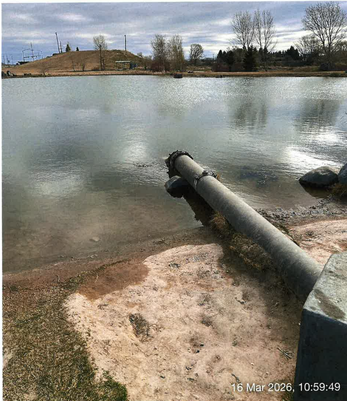
Pipe delivers water into the upper pond
