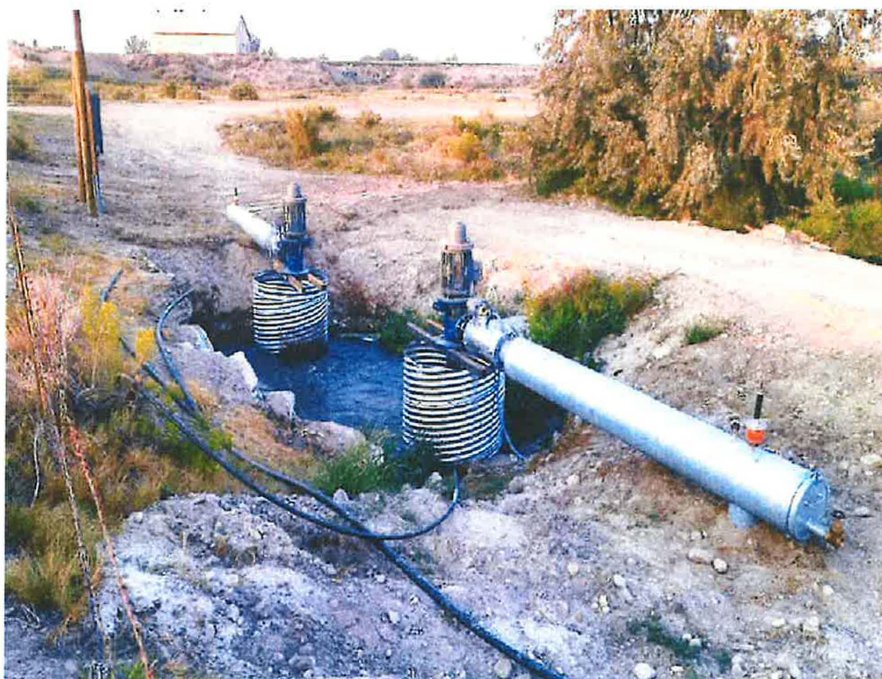
Photo 2-facing southwest- Pumps at the South Boise Drainage. Pump #1 is on the right, Pump #2 is on the left.
