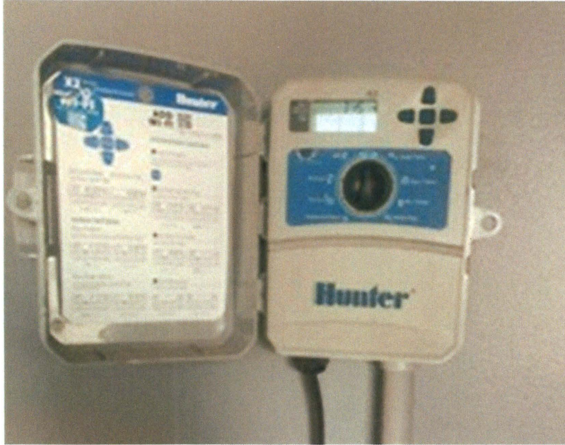
Figure 4 Control panel, photo provided by water permit owner.
