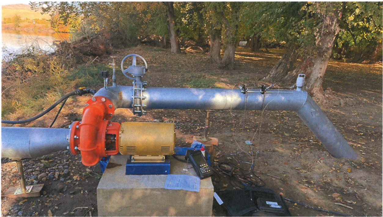
Figure 3 Point of diversion from Snake River with closed conduit flow meter attached. Photo includes Baldor Reliance pump motor and straight length conduit.
