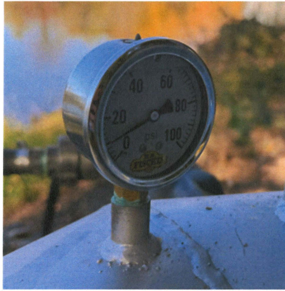
Figure 4 Pressure gage reading 10psi at the time of the field exam.
