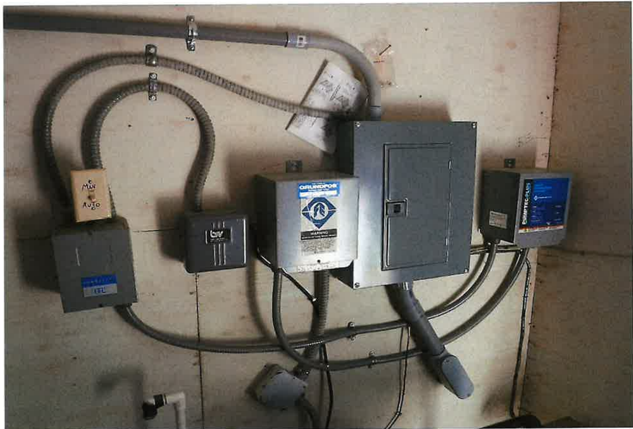
DIVERTING WORKS – INCLUDE 2 – HP GRUNDFOS PUMP WITH FRANKLIN ELECTRIC PUMP MOTOR
