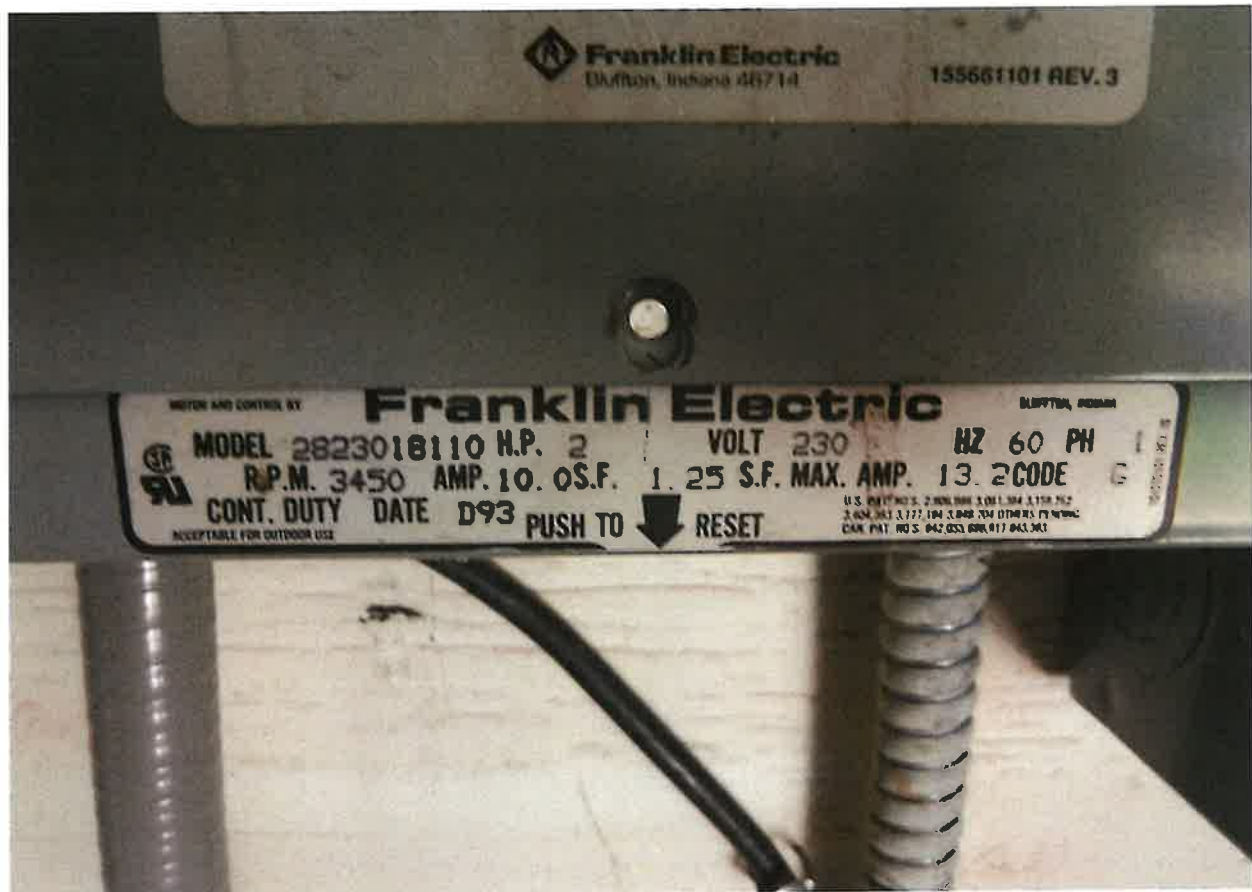
POD – FRANKLIN ELECTRIC 2 HP PUMP MOTOR MODEL 2823018110
