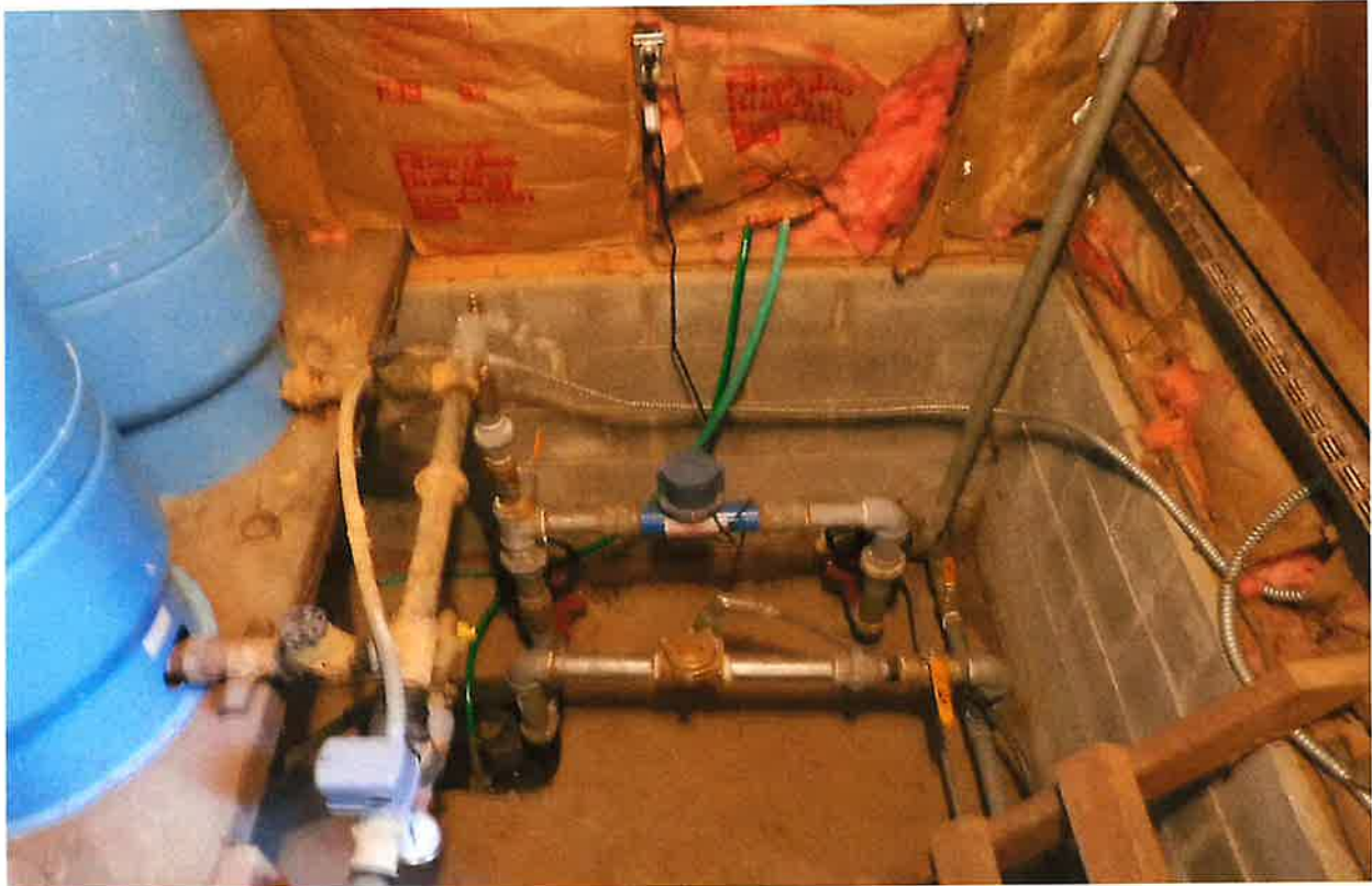
WATER SYSTEM HAS A SINGLE CROSS CONNECTION WITH OUTLET WATER ASSN MUNICIPAL WATER SYSTEM (BACK-UP TO THIS SYSTEM)
