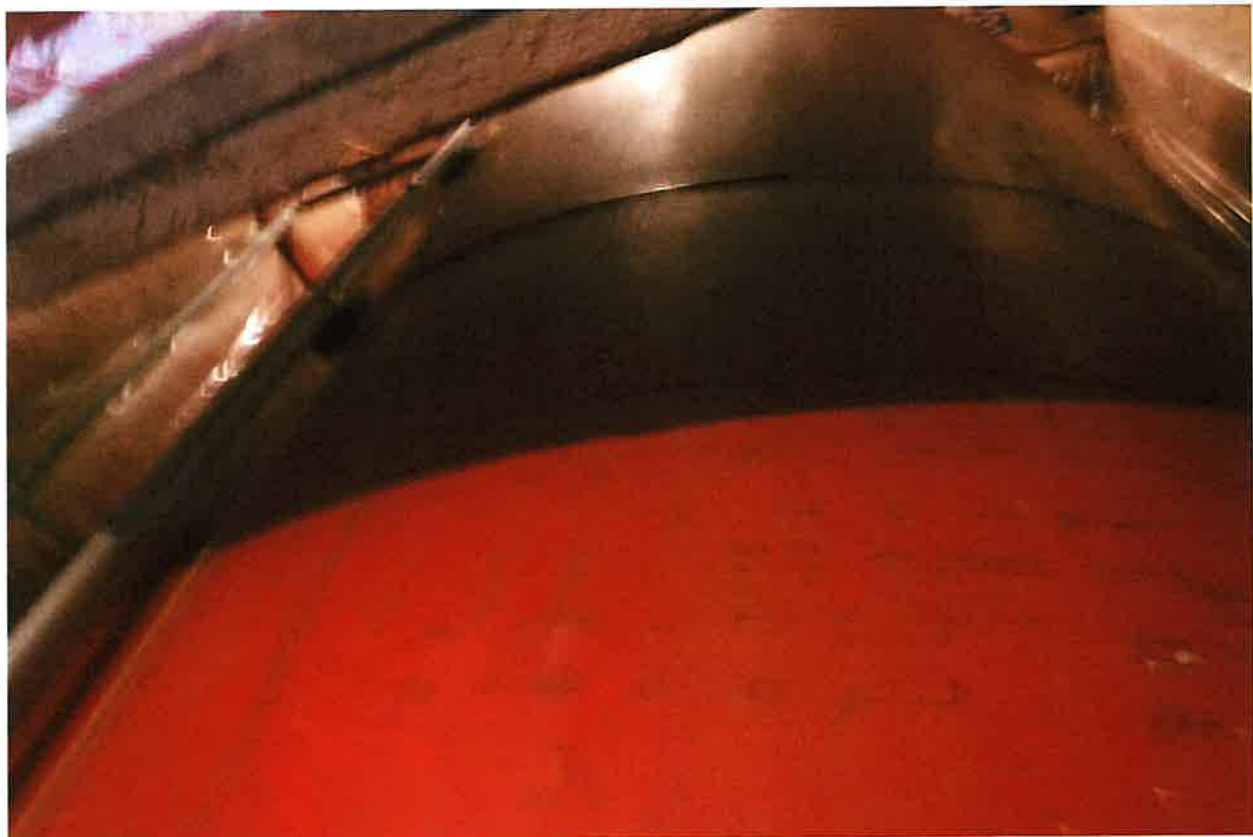
CONVEYANCE SYSTEM – INCLUDES 6,000 GAL STORAGE RESERVOIR
