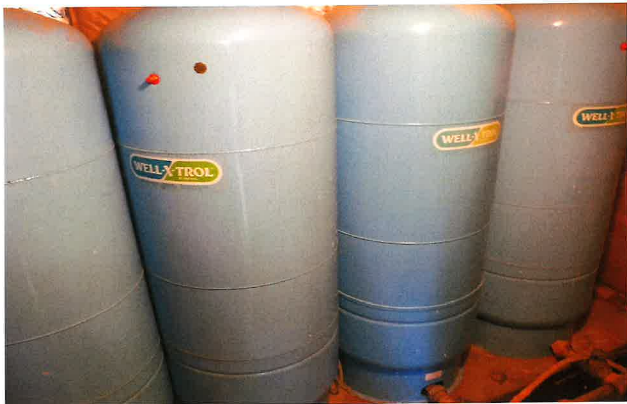
FOUR PRESSURE TANKS SUPPORT DOMESTIC SERVICES TO 36 HOMES
