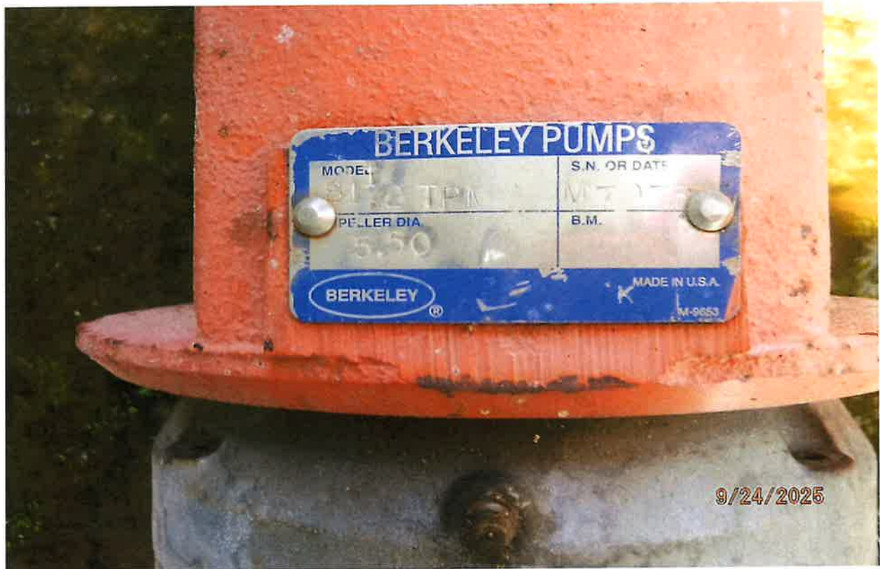
DIVERTING WORKS – 5 HP BERKELEY PUMP, S/N M7975 WITH 2-INCH DISCHARGE
