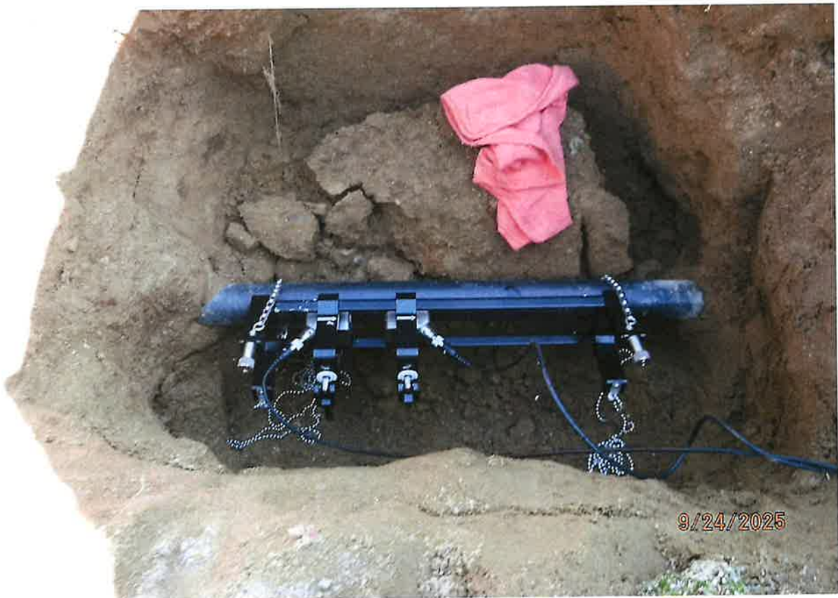
ILLUSTRATION OF FLOWMETER INSTALLATION USED TO MEASURE PUMP CAPACITY AT TIME OF FIELD EXAM
