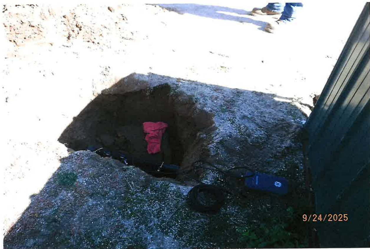
PUMP CAPACITY FLOW MEASUREMENT TAKEN NEAR PUMP STATION ATTACHING GE PT900 FLOWMETER TO SECTION OF 2-INCH MAIN PIPELINE
