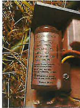
Pump starter with capacity info
