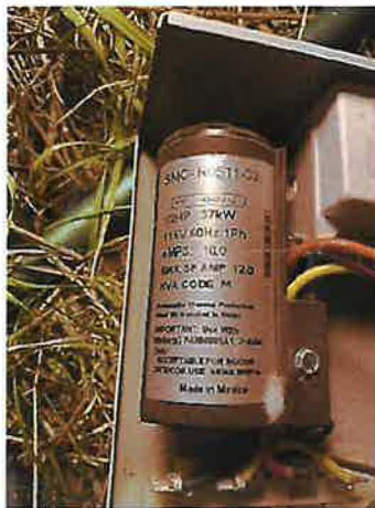
Pump starter with capacity info
