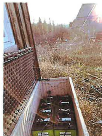
Solar batteries and panels that power the pump
