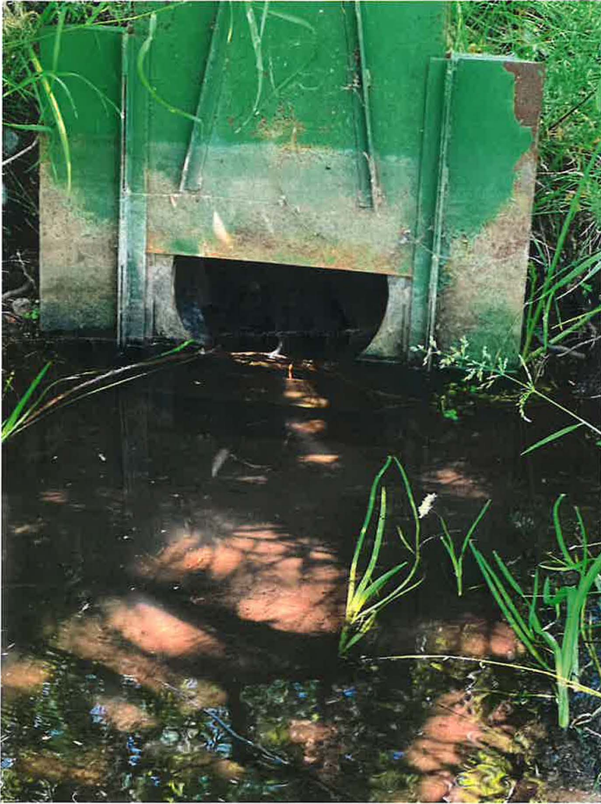
Lockable device providing the watermaster suitable control of the diversion, located upstream of the pump intake.
