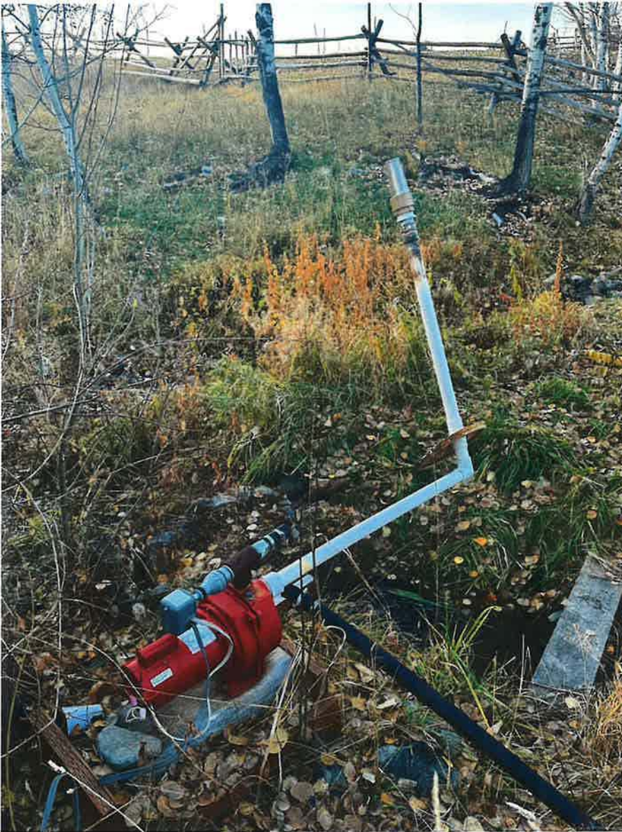
Pump and fish screen attached to the inlet in accordance with IDFG permit conditions
