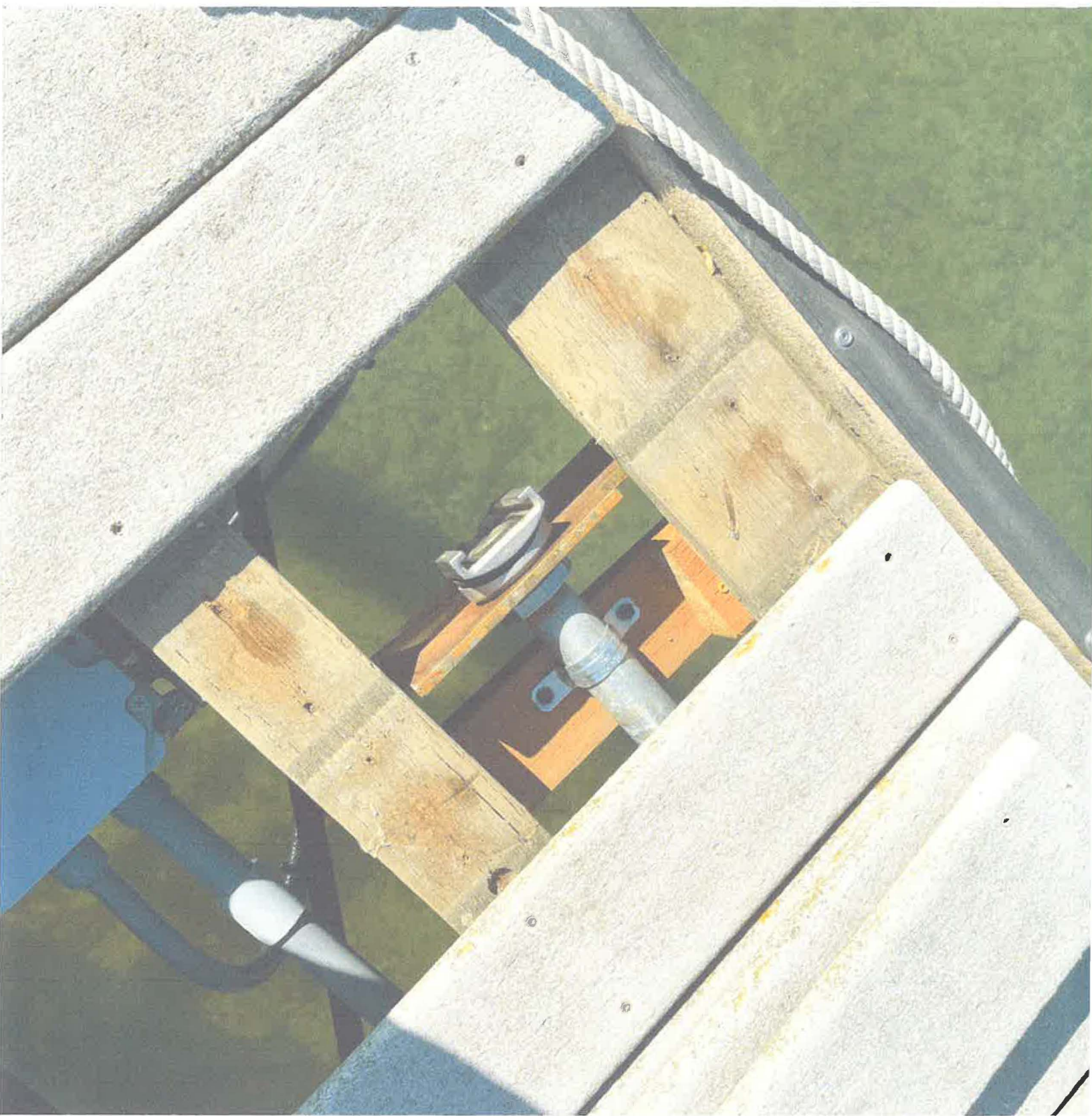
p.t. Less connection for Pump At End of Dock
