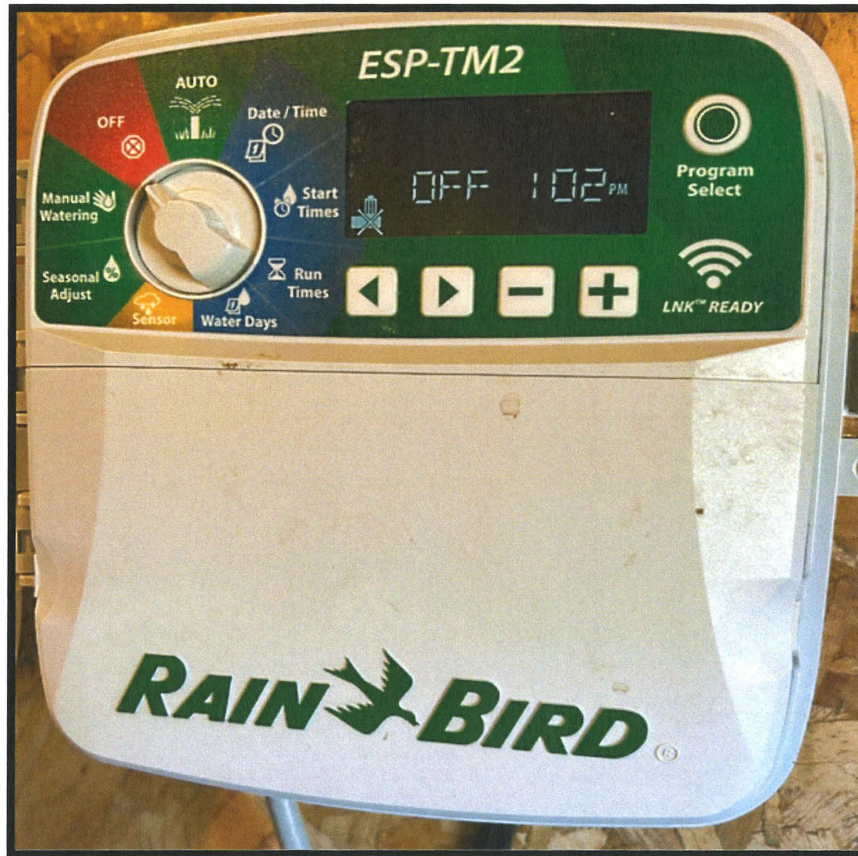
Photo 6- Irrigation control panel- on northwest wall of pump house.
