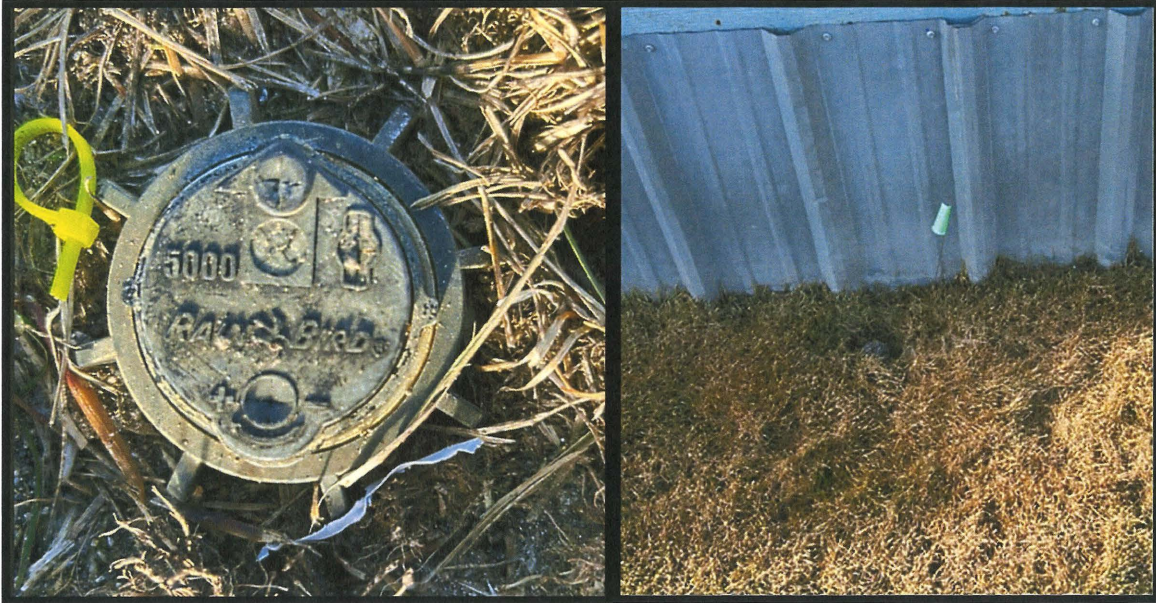
Photo 14-(above-left) Rainbird sprinkler heads found through out the irrigated areas. Photo 15 (above-right) Rainbird head alongside a home in the NE irrigated area.
