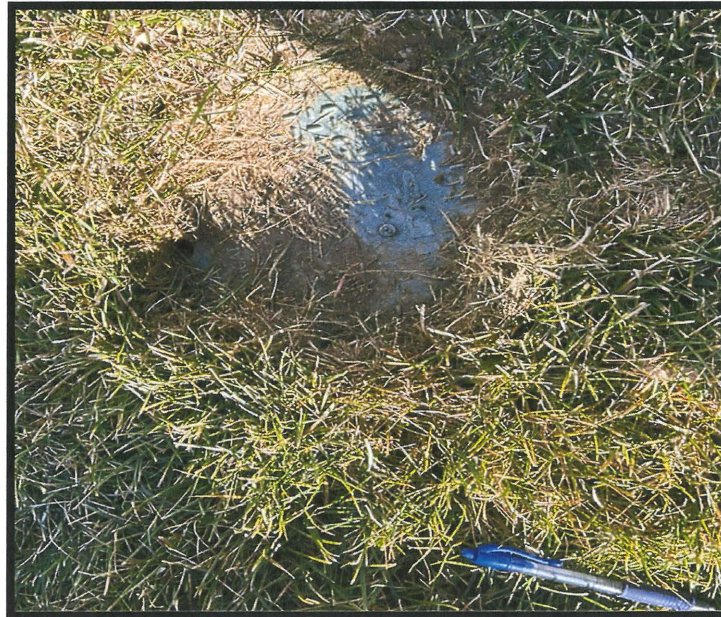
Photo 13- Control Valve at the SE end in irrigated area between rows of homes.
