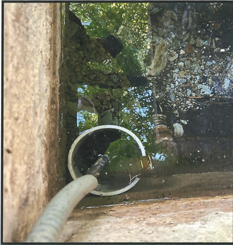
Photo 7- 6" PVC in lower left corner of the spring box, both diversion lines visible. Black line exiting to the upper left of the spring box is diversion to permit holder's home. The grey line exiting the lower left of the spring box surrounds the black poly and power cord associated with diverting water for WR 74-16009 (visible in photo 6).
