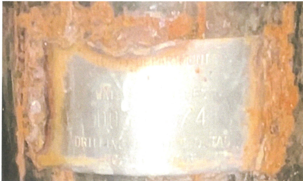
Figure 17 Metal tag for well 3, D0046574.
