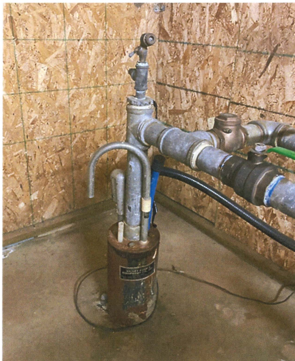
Figure 20 Well 4 head. No metal tag was available.
