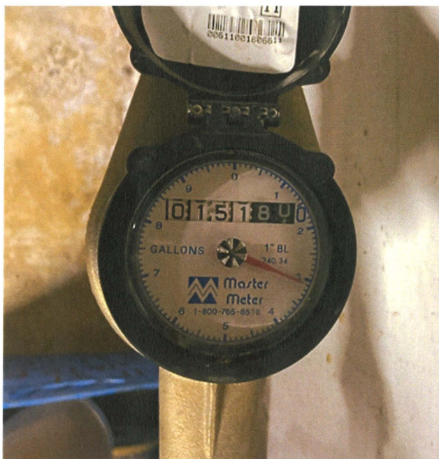
Figure 15 Lodge flow meter. All water utilized within the lodge including restaurant, bar, and public restrooms should be accounted for by this meter.
