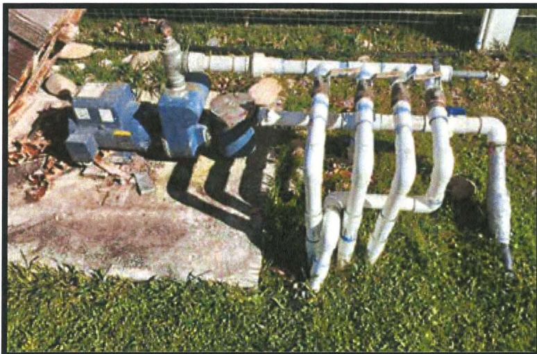
Photo 6- A Berkeley 5 Hp self priming centrifugal pump connected to a manifold for distribution of water throughout the irrigation from storage POU (image from FE for 63-34114).
