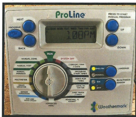
Photo 9- Controller for front Island irrigation with 4 zones, driplines for trees and small umbrella popups for small bushes in landscaped beds
