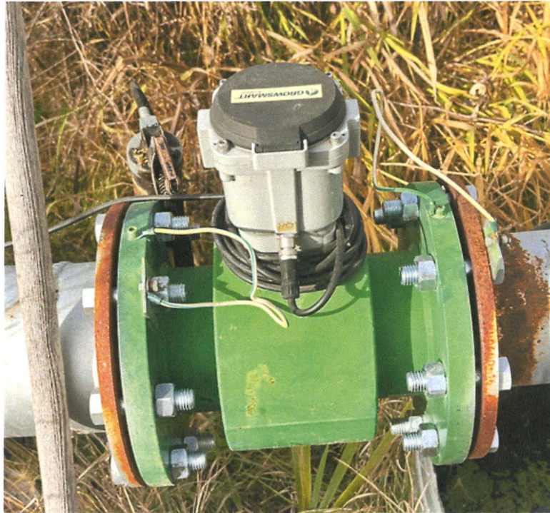
Figure 5 Growsmart by Lindsay Brand flow meter installed to the point of diversion.
