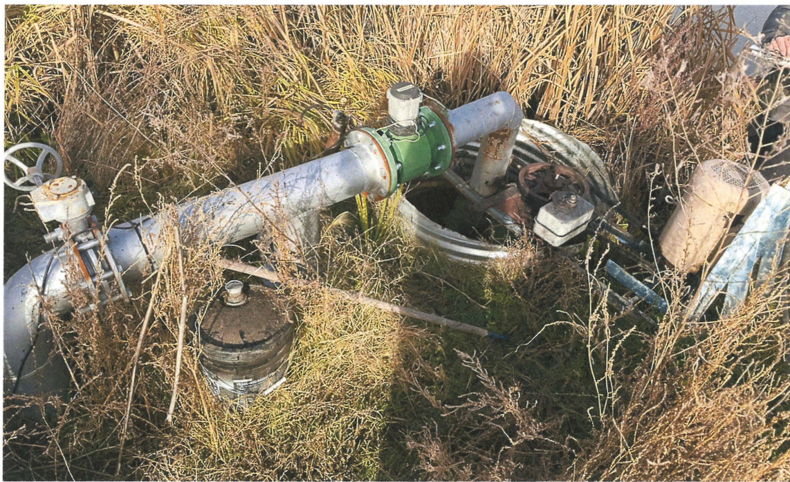
Figure 4 Point of diversion including 5hp pump and flow meter.
