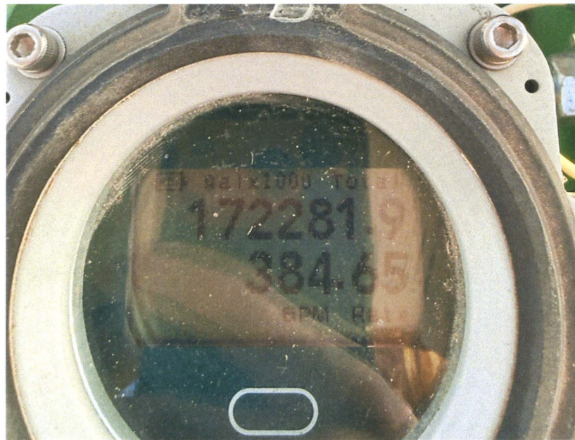
Figure 6 Flow meter reading collected at the time of the field exam, showing a diversion rate of 384.65 GMP, or 0.78cfs.
