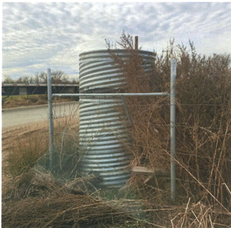
Figure 10 Riser associated with 6.5-acre field, located on the Southeast corner of field 1.
