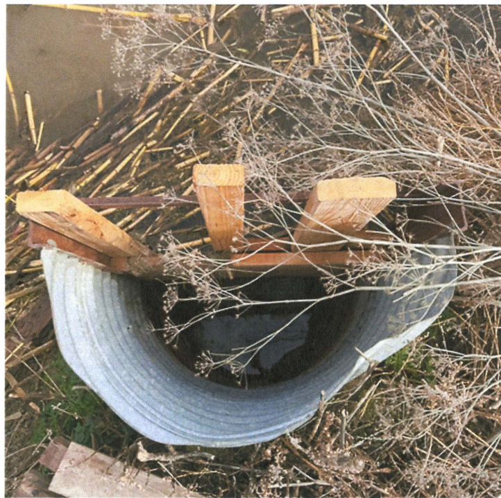
Figure 14 Outlet located on West end of field 2.
