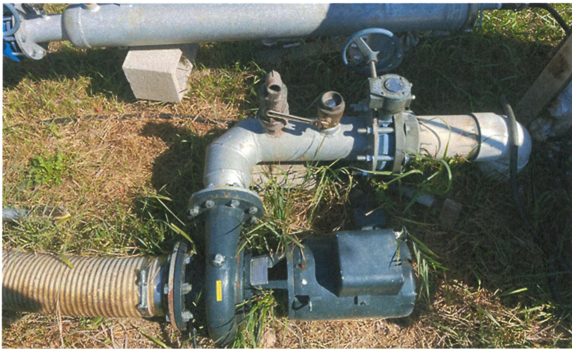
Figure 2 Baldor Reliance 5hp pump used to divert storage water.
