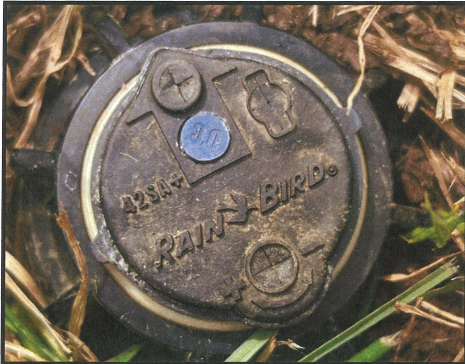
Photo 22- Rain Bird rotary sprinkler heads found throughout the lawn surrounding the permit holder's home.
