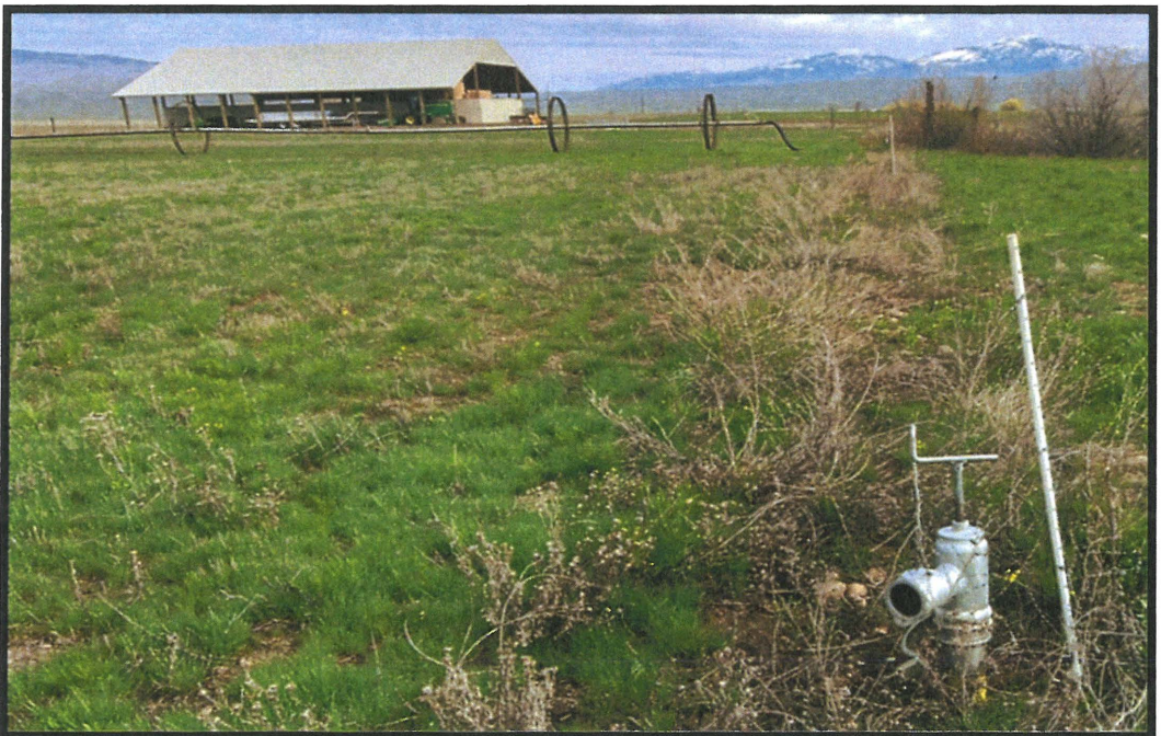
Photo 14- A row of 4" risers in the field north of the driveway and west of the home. Each is marked with a white rod. 4" flex line is used to connect the wheel line at each riser. The pond is visible in the upper right corner of the image.
