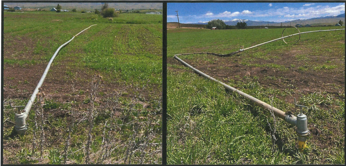
Photos 9 &10 – Standing along the west extent of the POU facing east. The handline and norther wheel line are connected to the row of risers.
