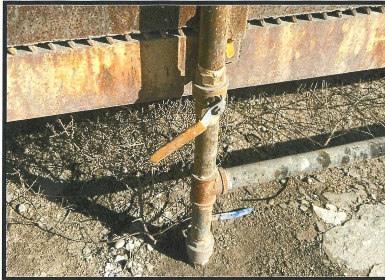
Photo 22- Hand valve for manually filling the barrel of mixers using the fill pipe (same on either side of the walk way).
