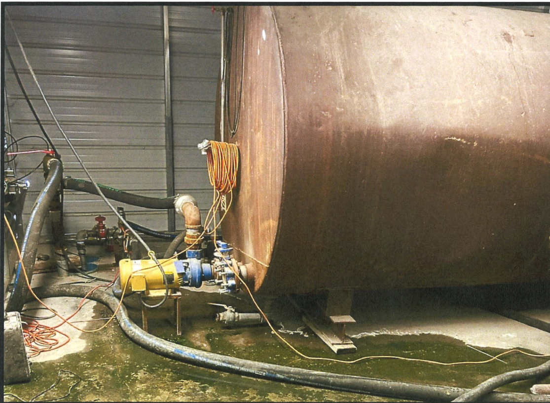
Photo 10- The boiler storage tank on the south end of the boiler room with its own 15Hp booster pump.
