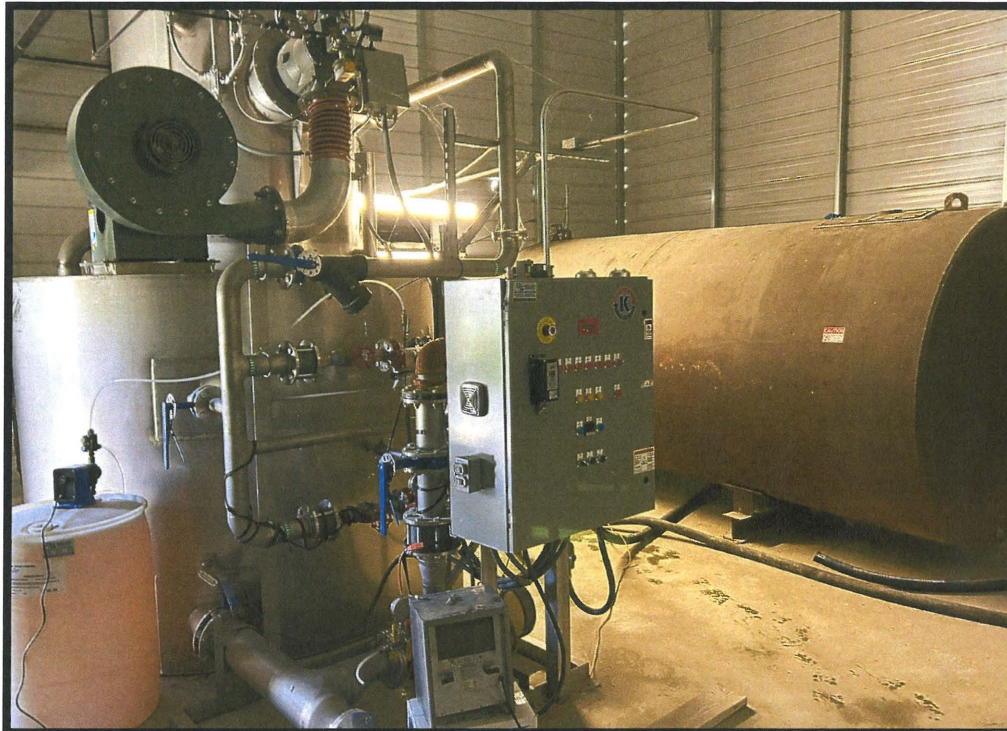
Photo 11- Water heater "boiler" and chiller system with intake manifold in image behind the control panel.
