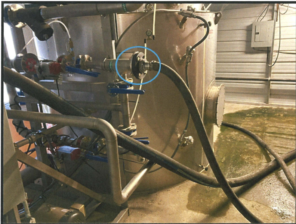
Photo 12- 2" flex line attached to the manifold (circled in blue). The servo actuated control valve can be seen to the left. The booster pump is in front of the manifold in the lower left of the image.
