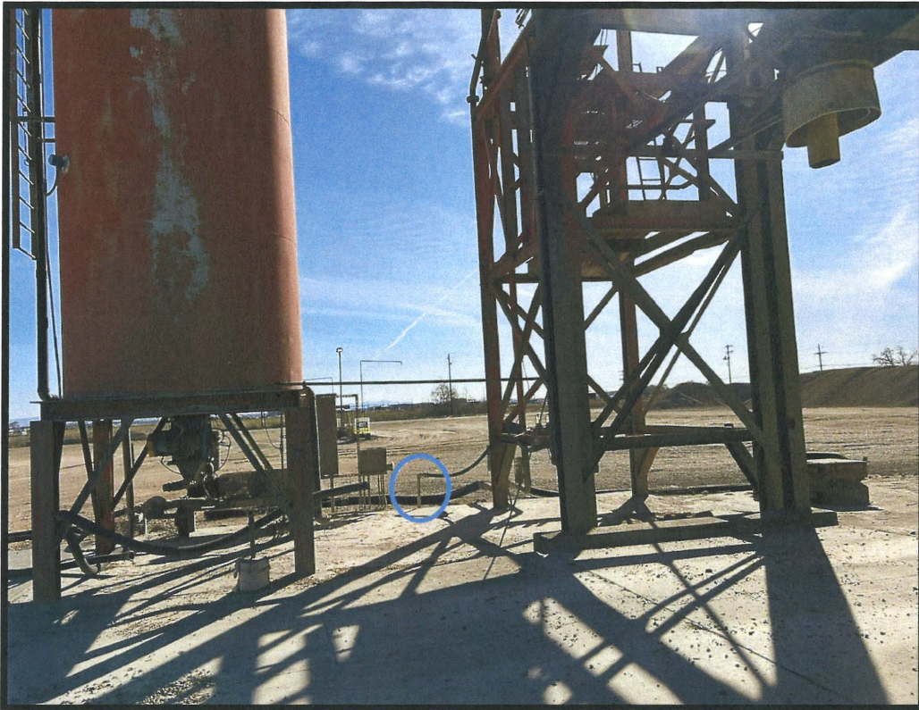
Photo 20- 2" flex line attached to the riser for the buried 2" galvanized pipe delivering water to the truck wash in the background.
