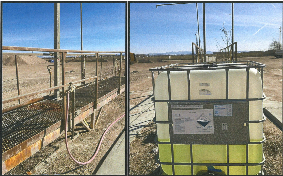
Photos 23 (left) Hose bibs on either side of the elevated walk way. Photo 24 (right) Hydrochloric acid for scrubbing and loosening hardened slurry off of truck barrels.
