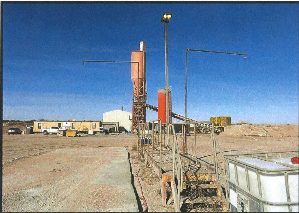
Photo 21- Facing west with the elevated walkway between the two truck wash stations in the foreground. The fill lines and hoses for cleaning trucks can be seen on either side.
