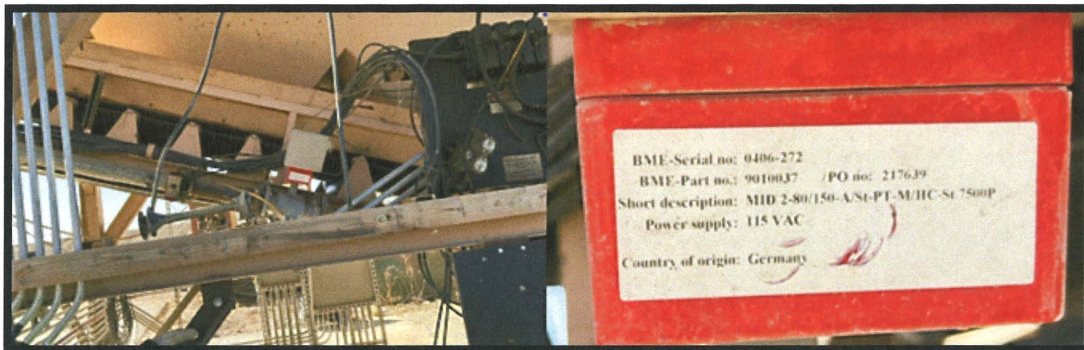
Photo 18- Control valve and flowmeter sensor box for metering water according to batch requirements.
