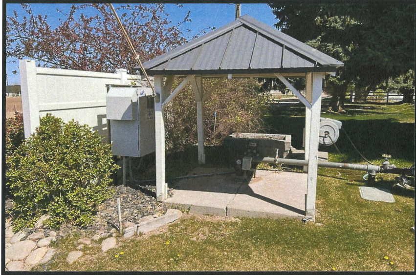
Photo 1- Irrigation system well head and VFD control panel located at the north end of the driveway to the home.
