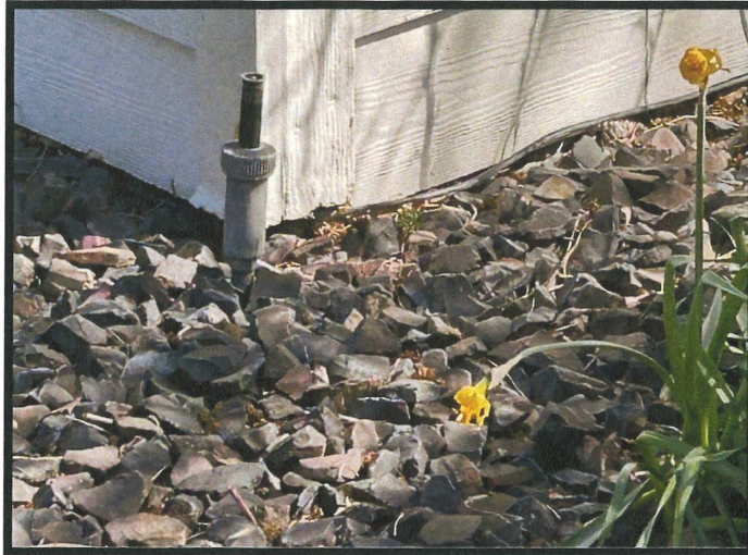
Photo 22- Umbrella popup sprinklers in landscaped bedding around the home.
