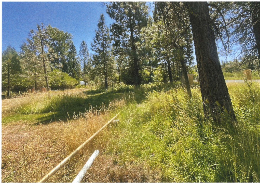
Figure 9 East facing photo of 4" mainline delivering water to east side of place of use.
