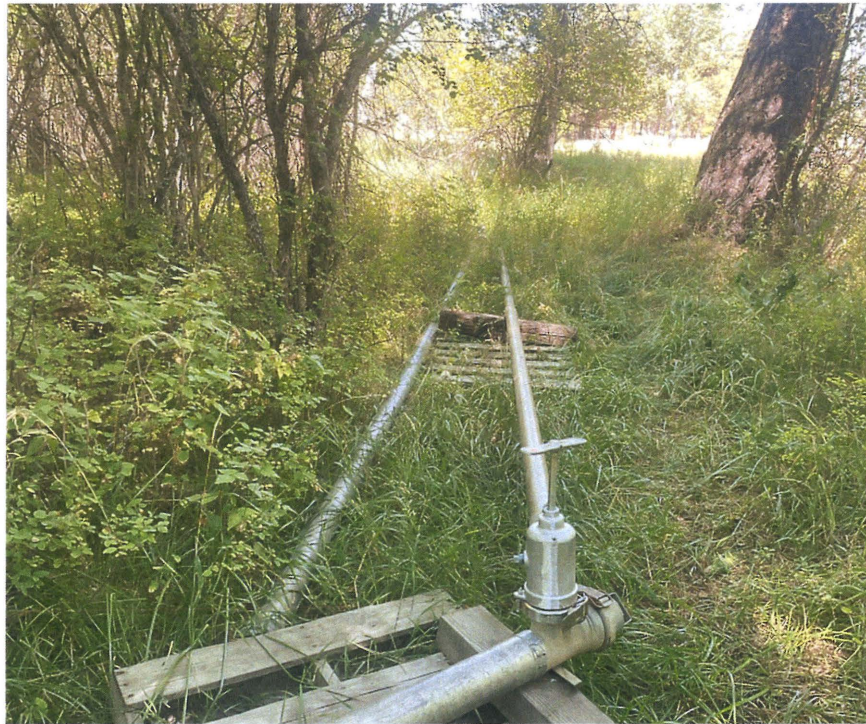
Figure 7 West facing photo of 4" mainline delivering water to west side of place of use.
