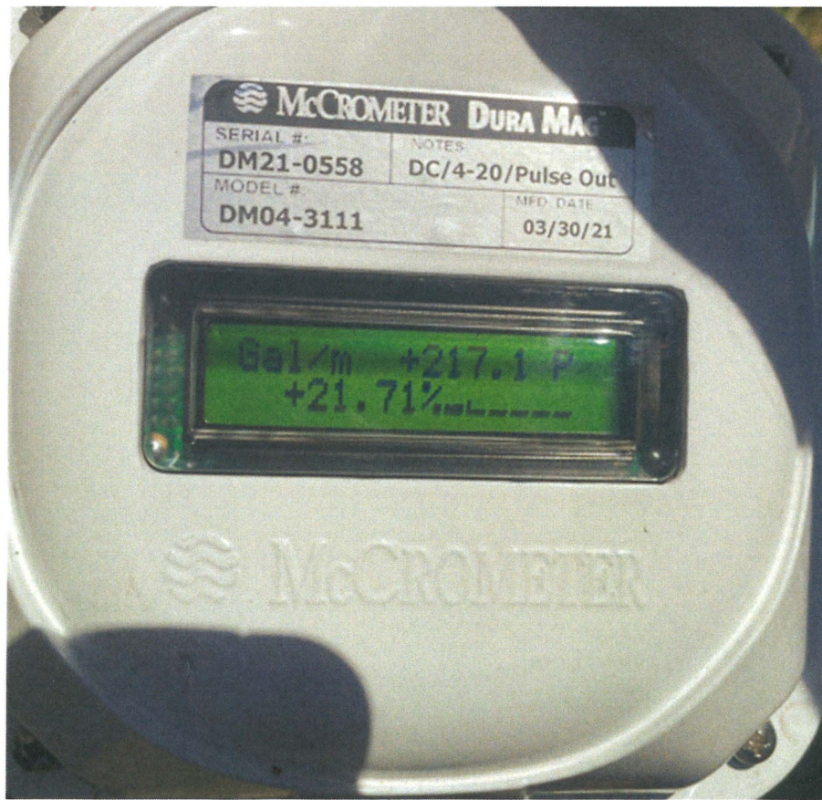
Figure 5 McCrometer Dura Mag flow meter installed to 65-23671 point of diversion.
