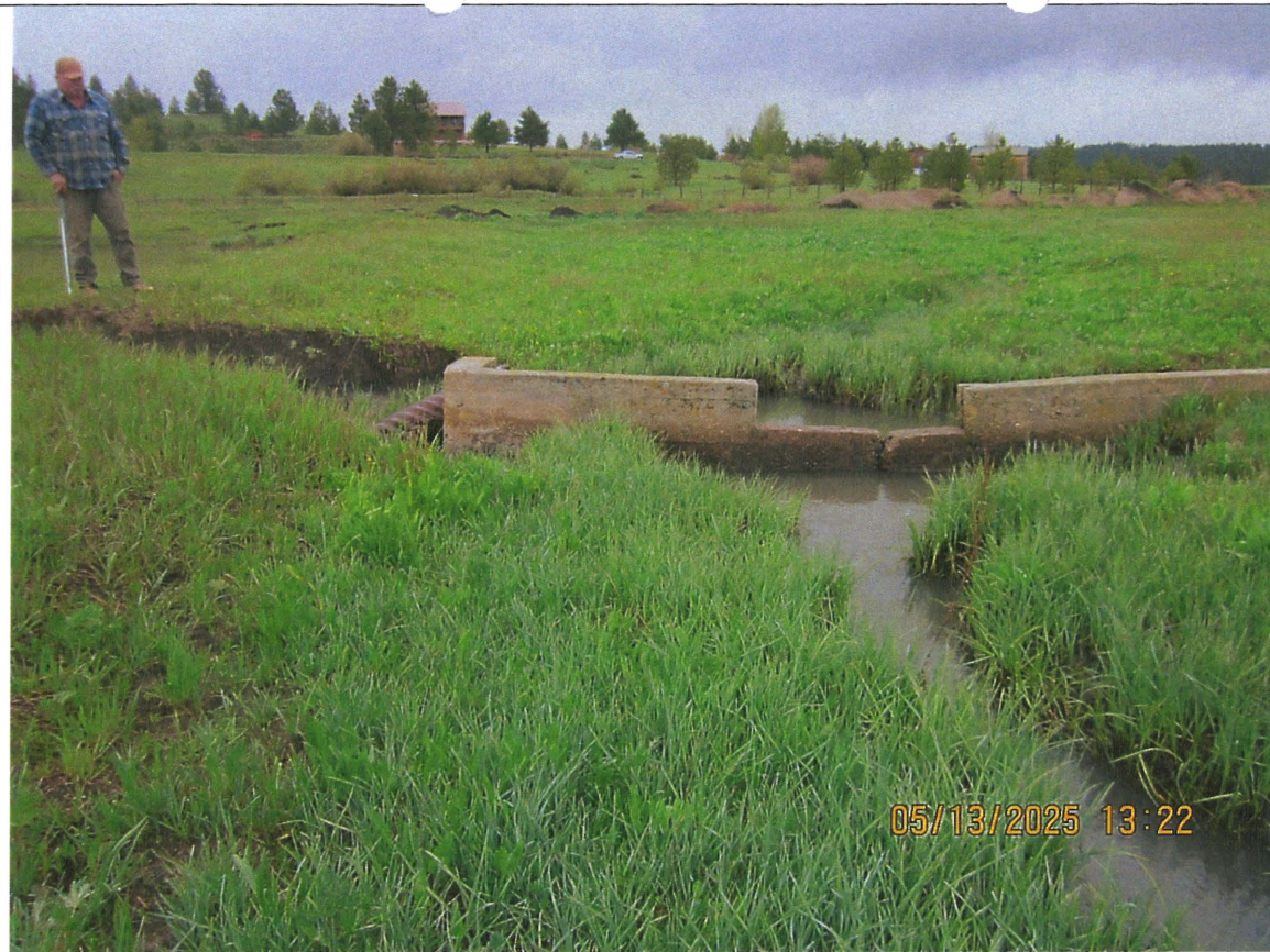
Figure 5. Water exiting the pond through a breach on the west side. The remains of a rectangular weir are in the foreground as water flows through and around it.
