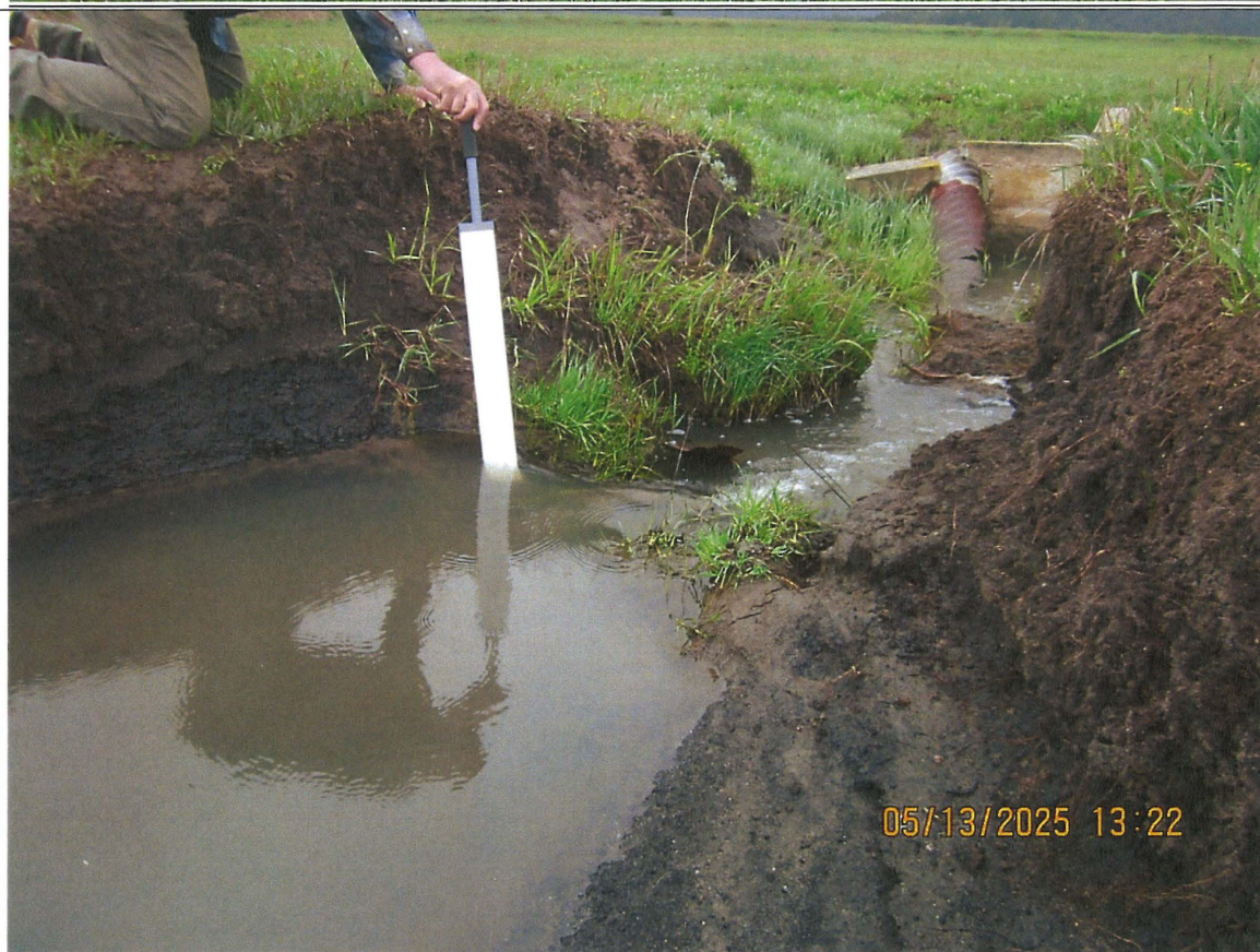
Figure 6. The breach in the pond where the water exits is about 115 feet south of the entry point.
