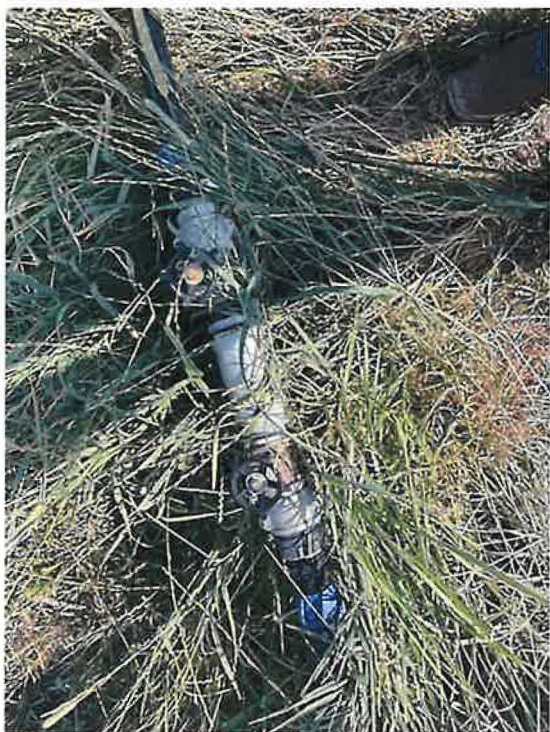
Figure 8. Photograph of riser in which two lines of k-pods consisting of 2 and 6 pods are connected and controlled by. Another riser to the south is used for another 5 pods but the permit holder could not use all 13 pods at the same time because the system could not handle it.
