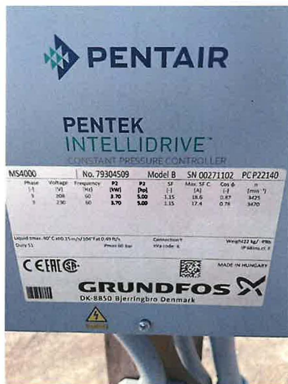
Figure 4. Photograph of variable speed specifications for the pump, found at the bottom of the pump control panel.
