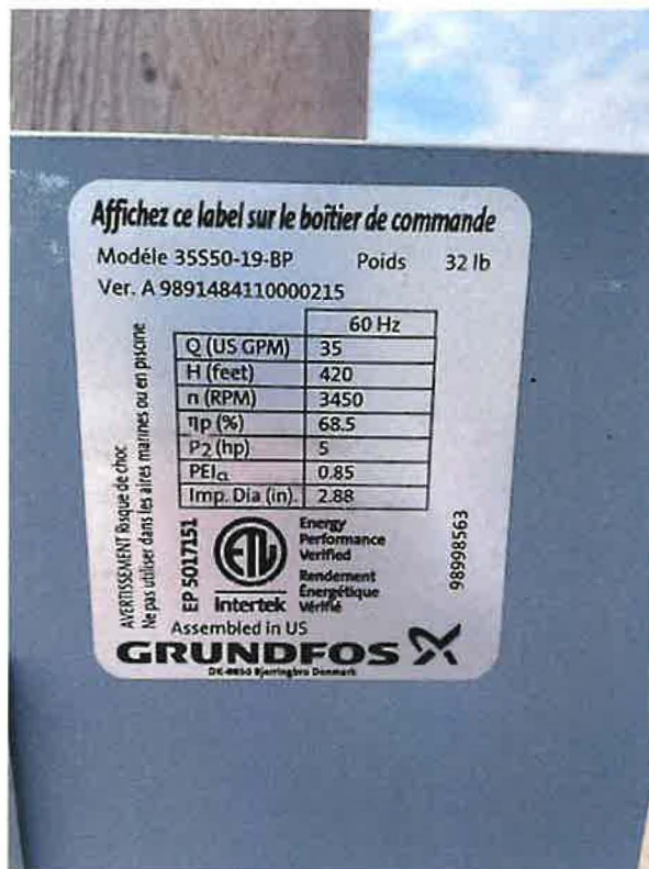
Figure 3. Photograph of pump specifications found to the right on the pump control panel.
