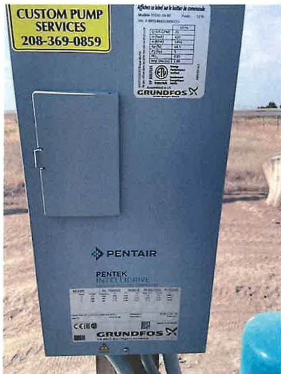
Figure 2. Photograph of pump control box with pump specifications.
