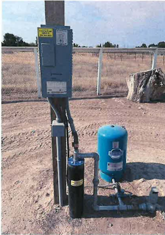
Figure 1. Photograph of the point of diversion and diversion system.
