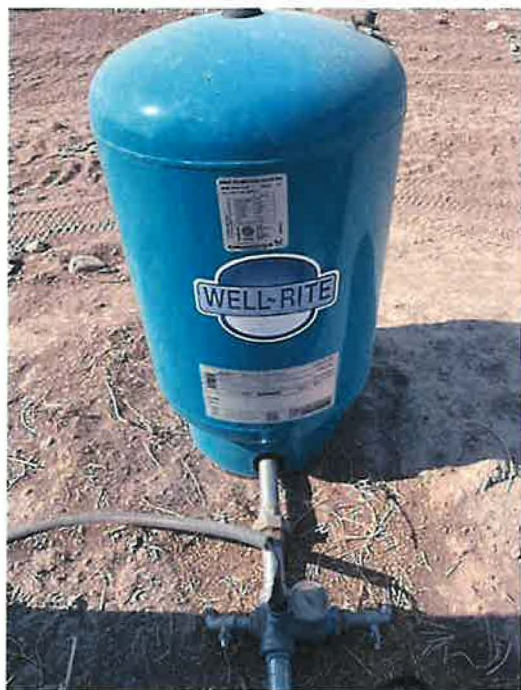
Figure 6. Photograph of pressure tank found the rear right from the well casing and control panel.
