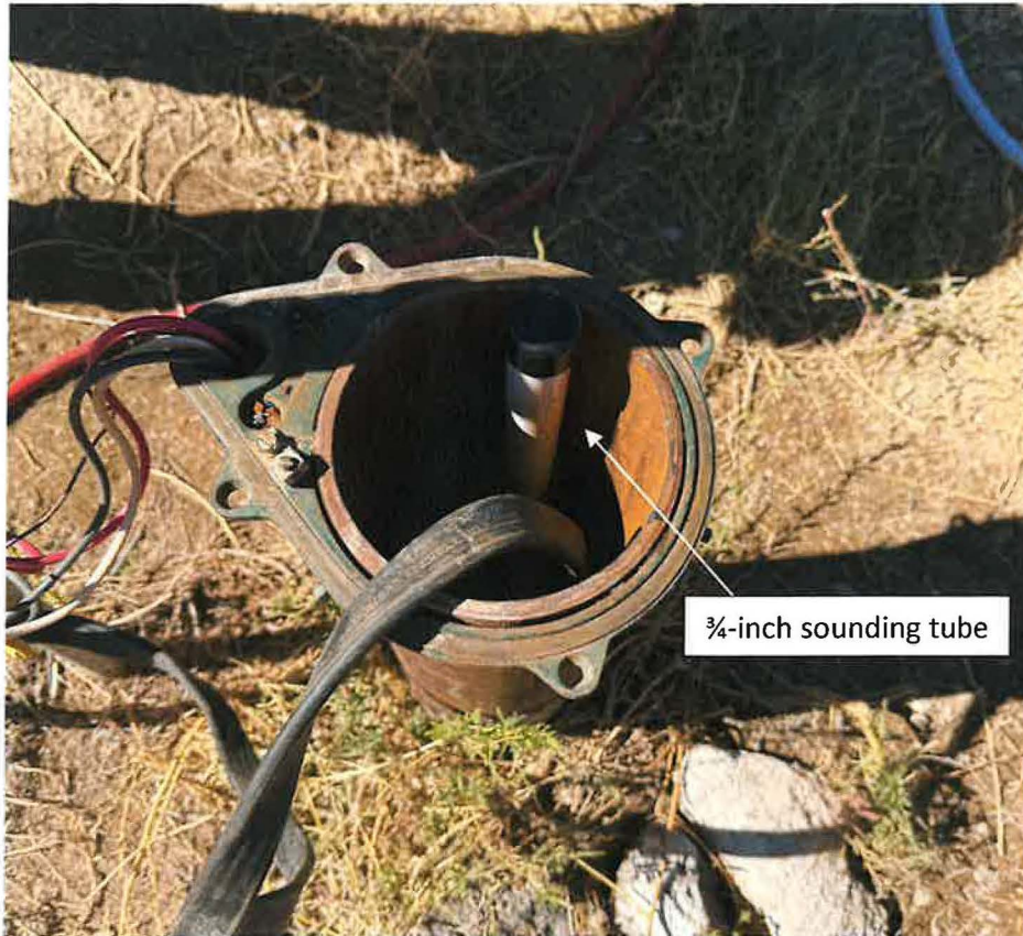
Figure 3. Sounding tube installed at well head per Condition 3 of the permit. Photo taken by permit owner and submitted 9/14/2025.
