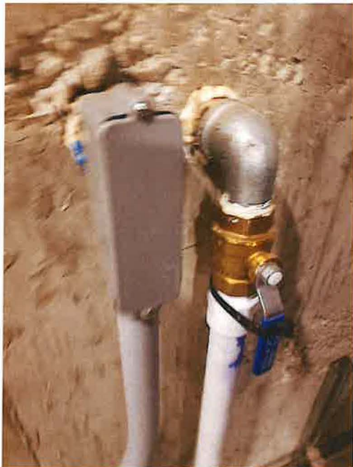
Distribution line into shop
