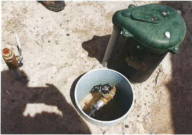
Well head and distribution pipe
