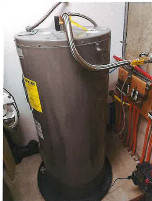
Hot water heater
