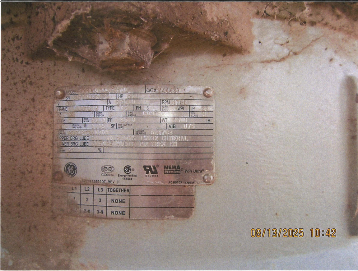
Figure 2. A single 200 hp GE pump model 5KS444DAJ6020A diverts water from the Snake River to a 12-inch diameter mainline.
