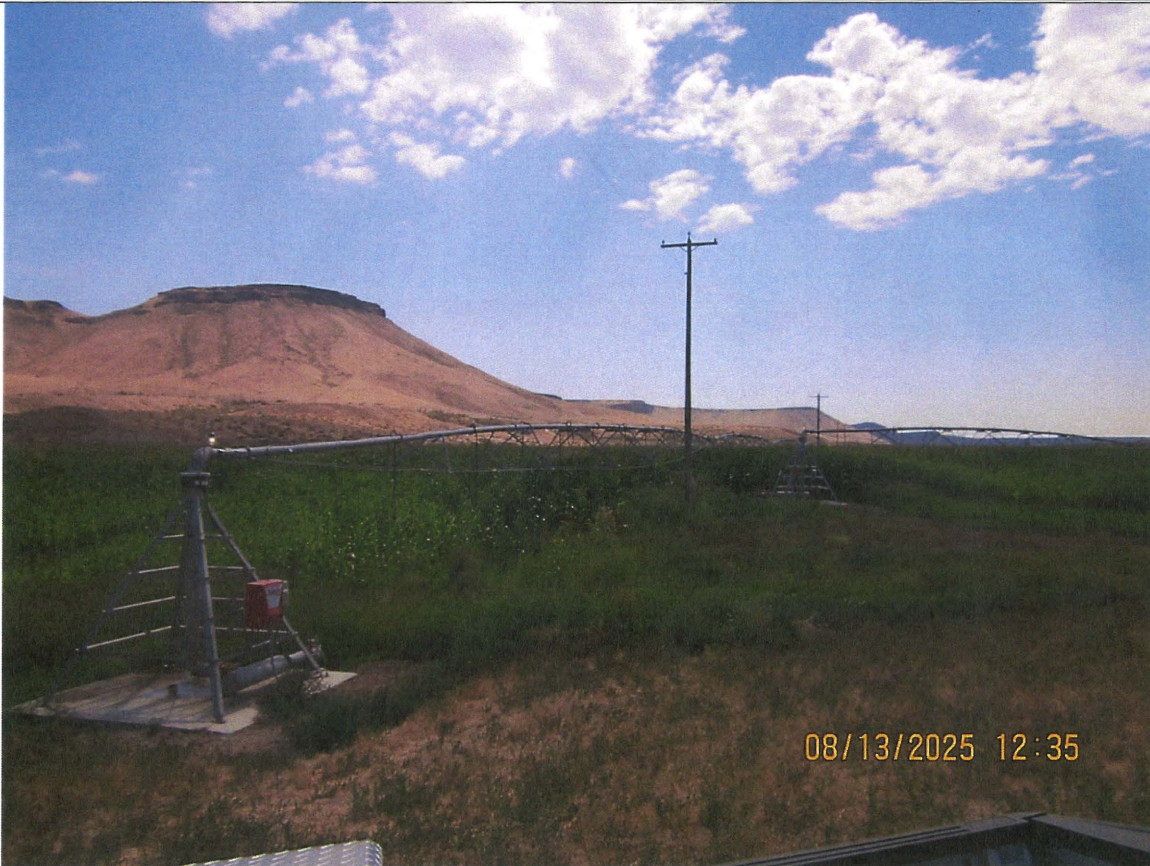
Figure 4. Pivot towers for pivots 44 and 46.
