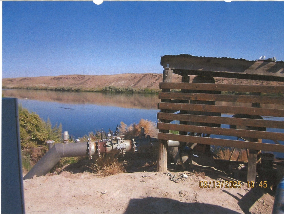
Figure 3. 12-inch mainline from pump at Snake River.
