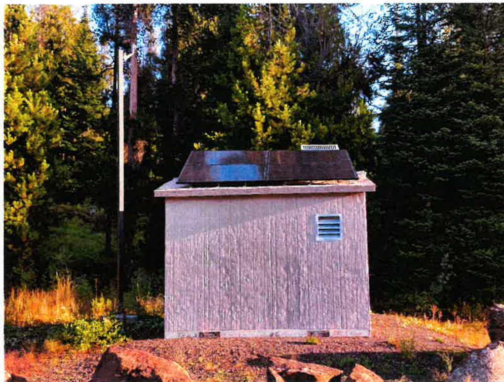
Figure 2: The pump house
