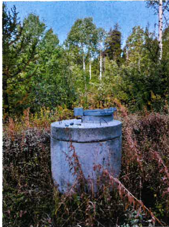
Figure 3: Top of 15,000 gallon storage tank
