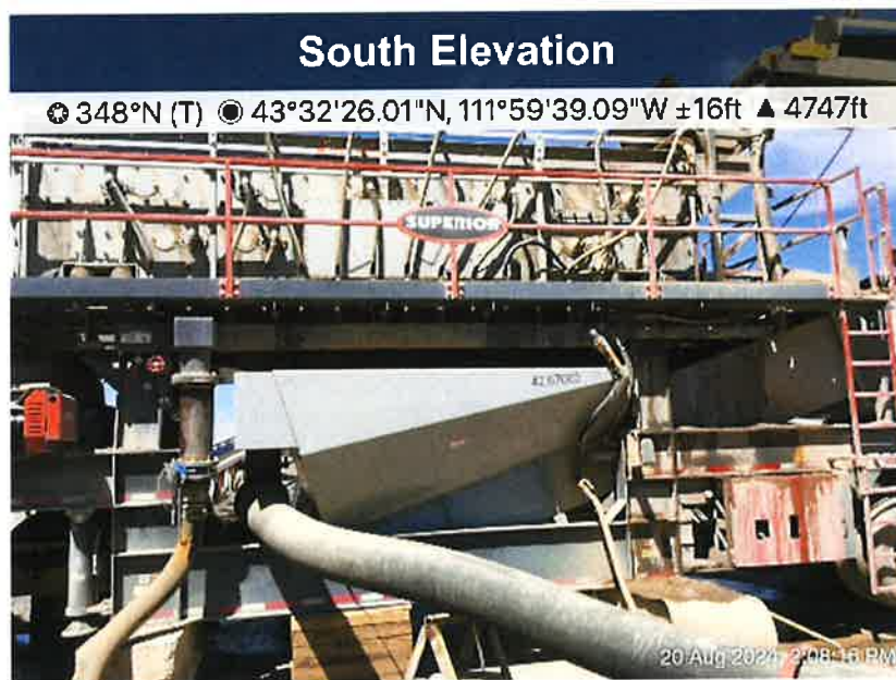
This is the new pump that sends water to wash station
