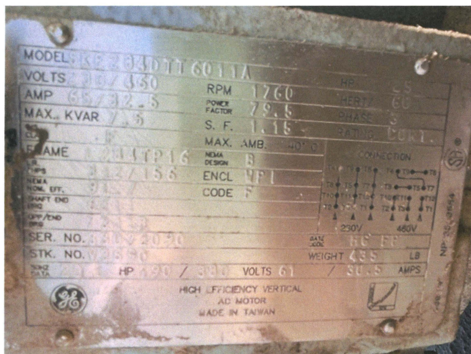
Figure 10 Pump tag for 25hp pump associated with storage pond.
