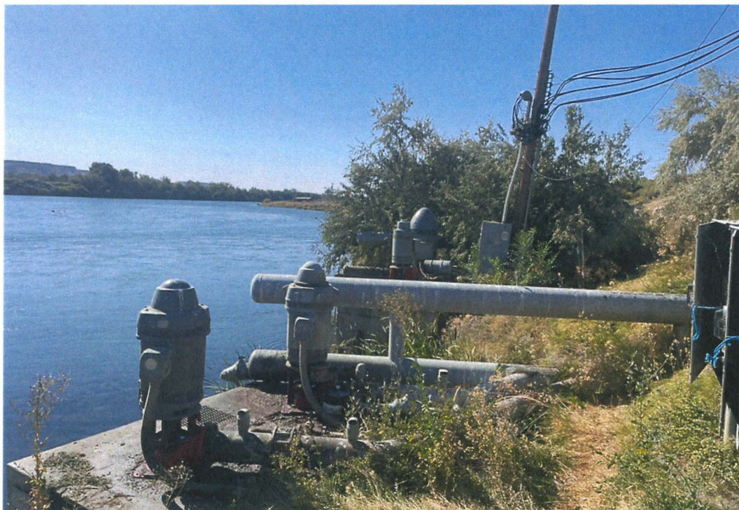
Figure 3 Point of diversion including four pumps to divert stockwater from the Snake River.
