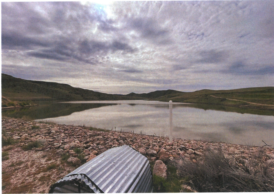
Figure 7 East facing photo taken from the point of diversion (hydraulic headgate). The photo includes a pipe vent, headgate cover, and western end of reservoir.
