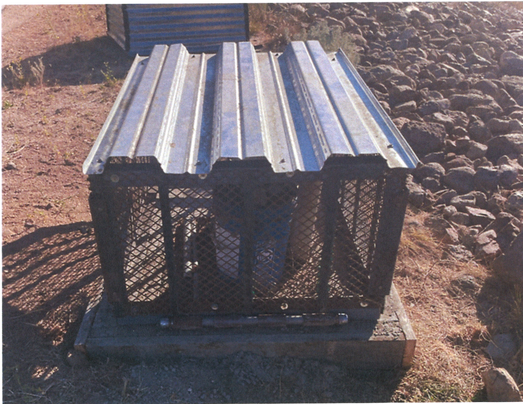
Figure 8 Photo of hydraulic headgate cover which was replaced after the field exam to install a lockable device.
