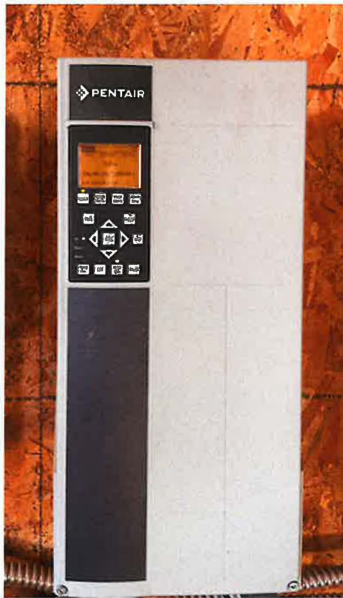
Figure 4 Control panel for well D0100371.
