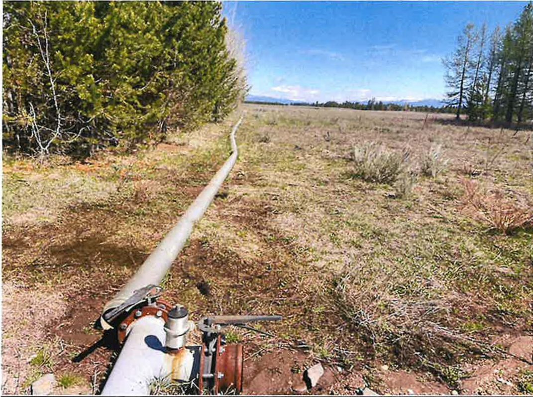
Figure 3 10" mainline that was used to deliver water to the irrigated place of use.
