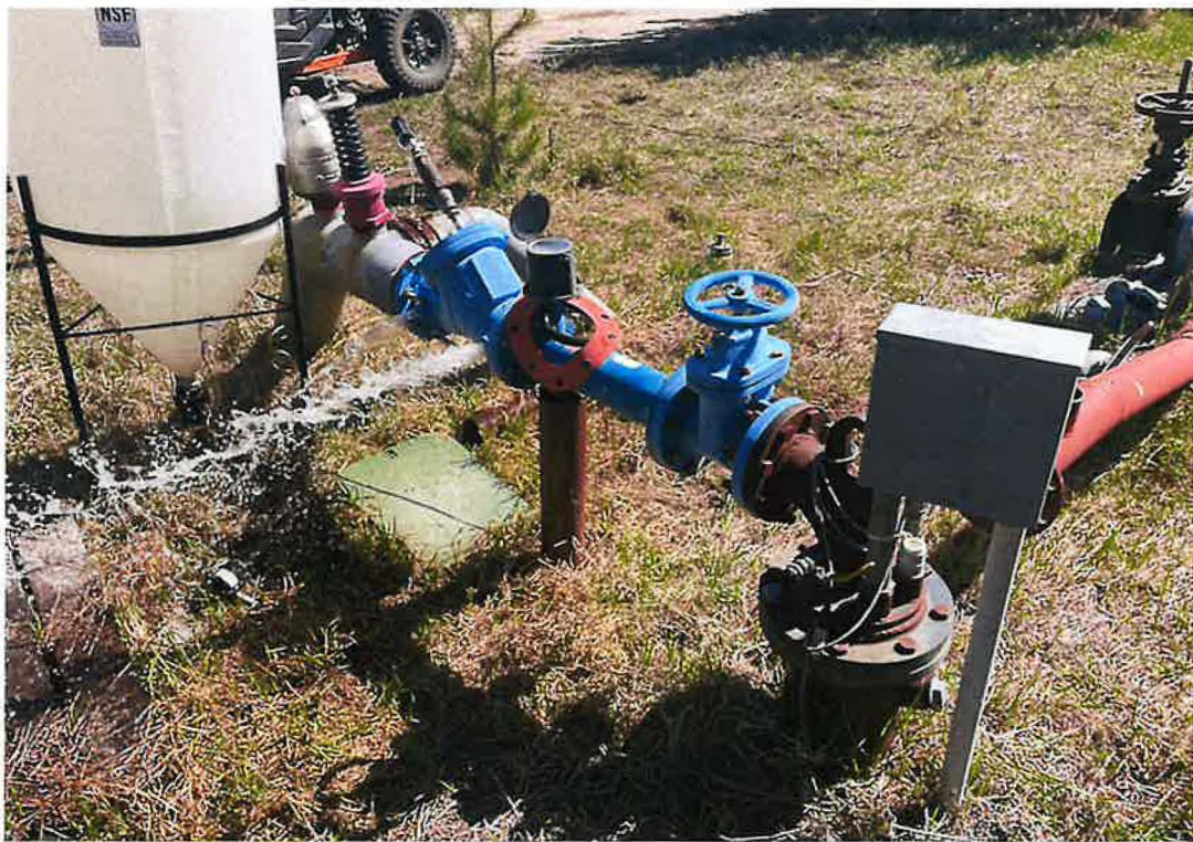
Figure 4 Point of diversion (well).
