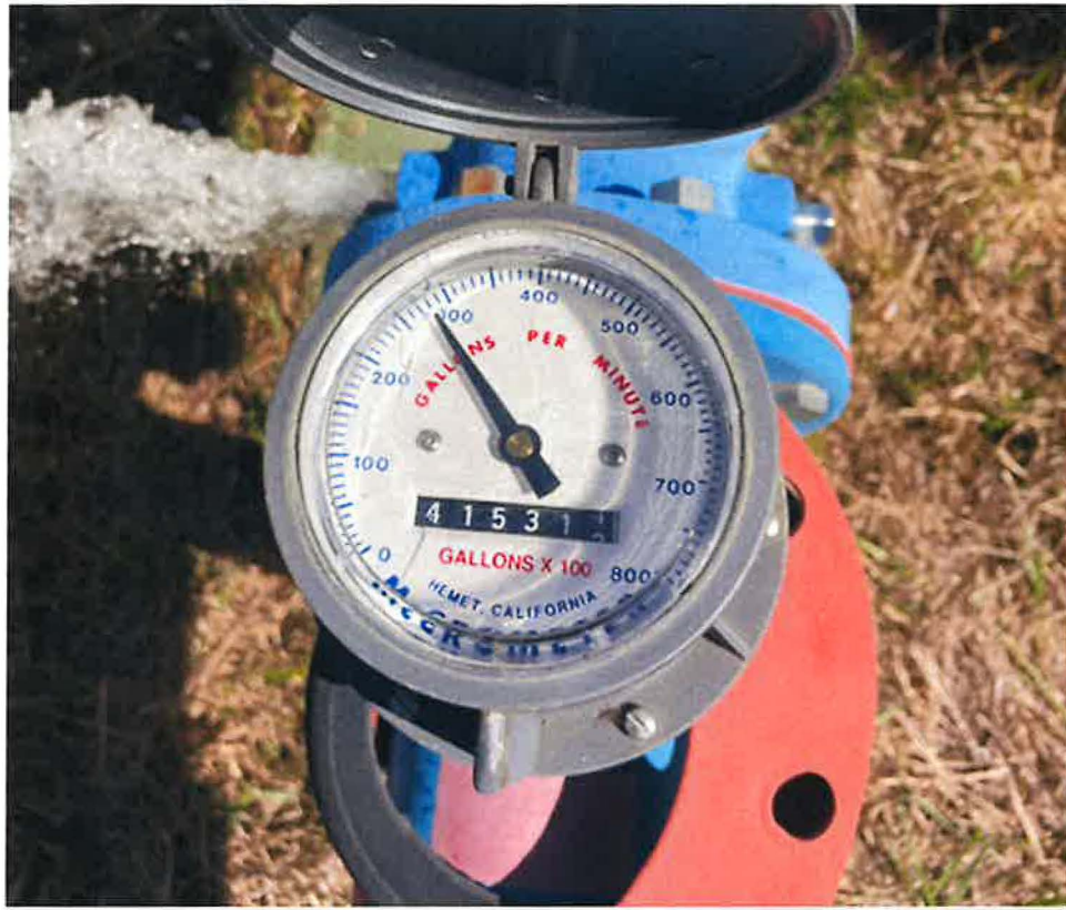
Figure 5 McCrometer flow meter installed to the irrigation system, near the well head. At the time of the field exam, the flow meter showed a current rate of 280 gpm.
