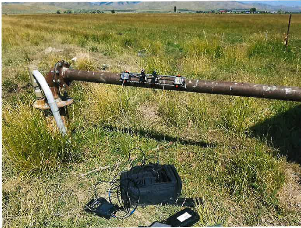
Ultrasonic flowmeter measurement conducted by Cooper Fritz
