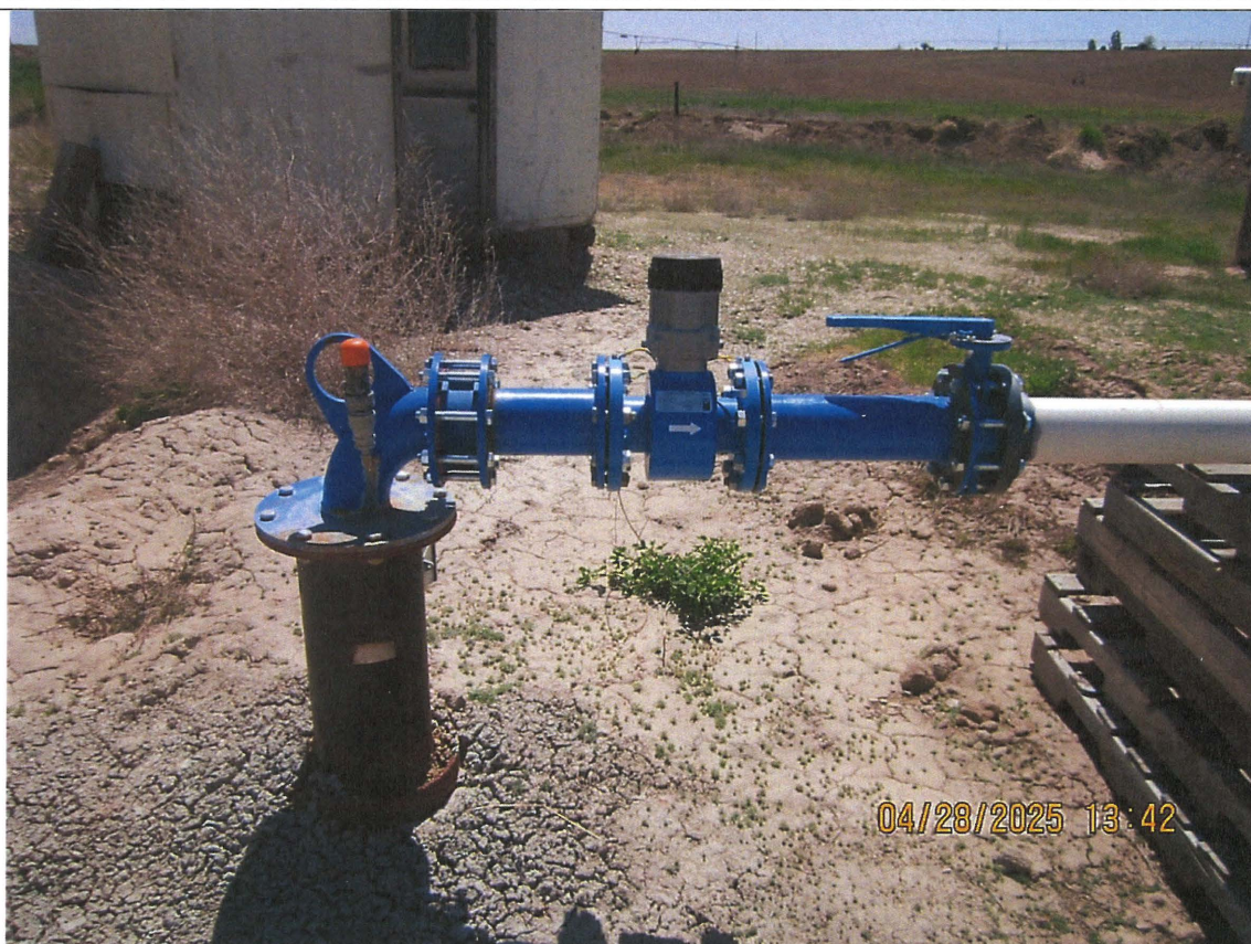
Figure 2. Well head and electromagnetic flowmeter from GloTech Corp.
