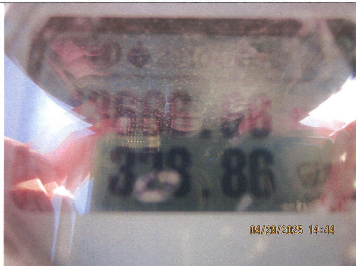
Figure 4. Flowmeter reading of 328.86 gpm.
