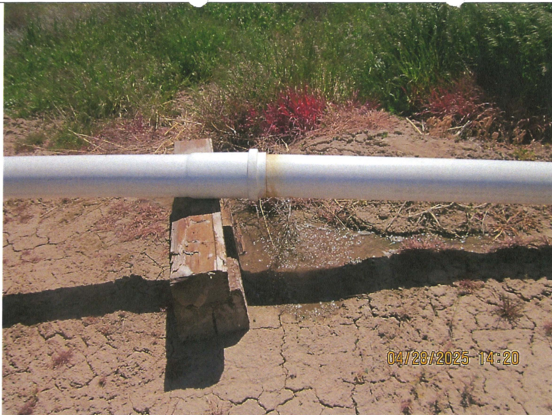
Figure 5. Leaks in line.
