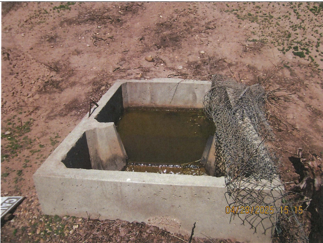
Figure 8. Measurement weir for surface water.
