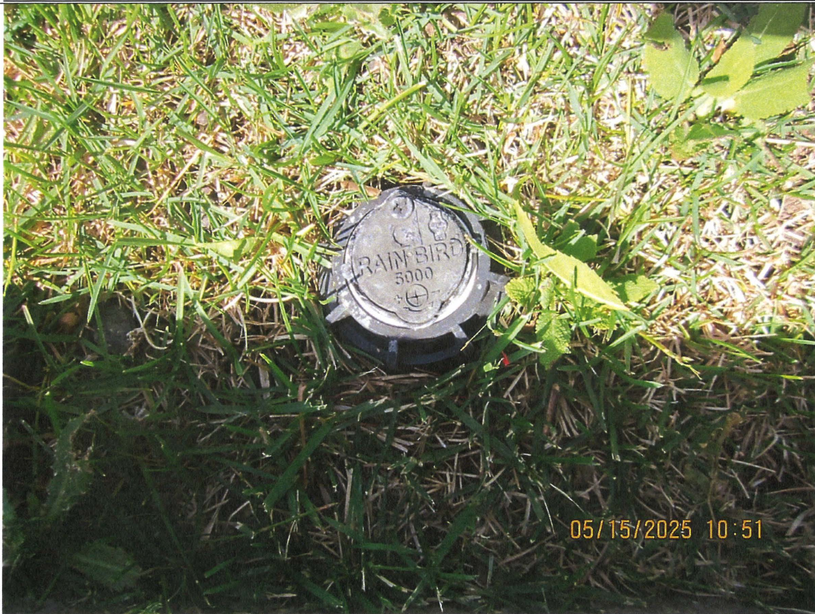
Figure 10. Rainbird 5000 sprinklers for lawn irrigation.
