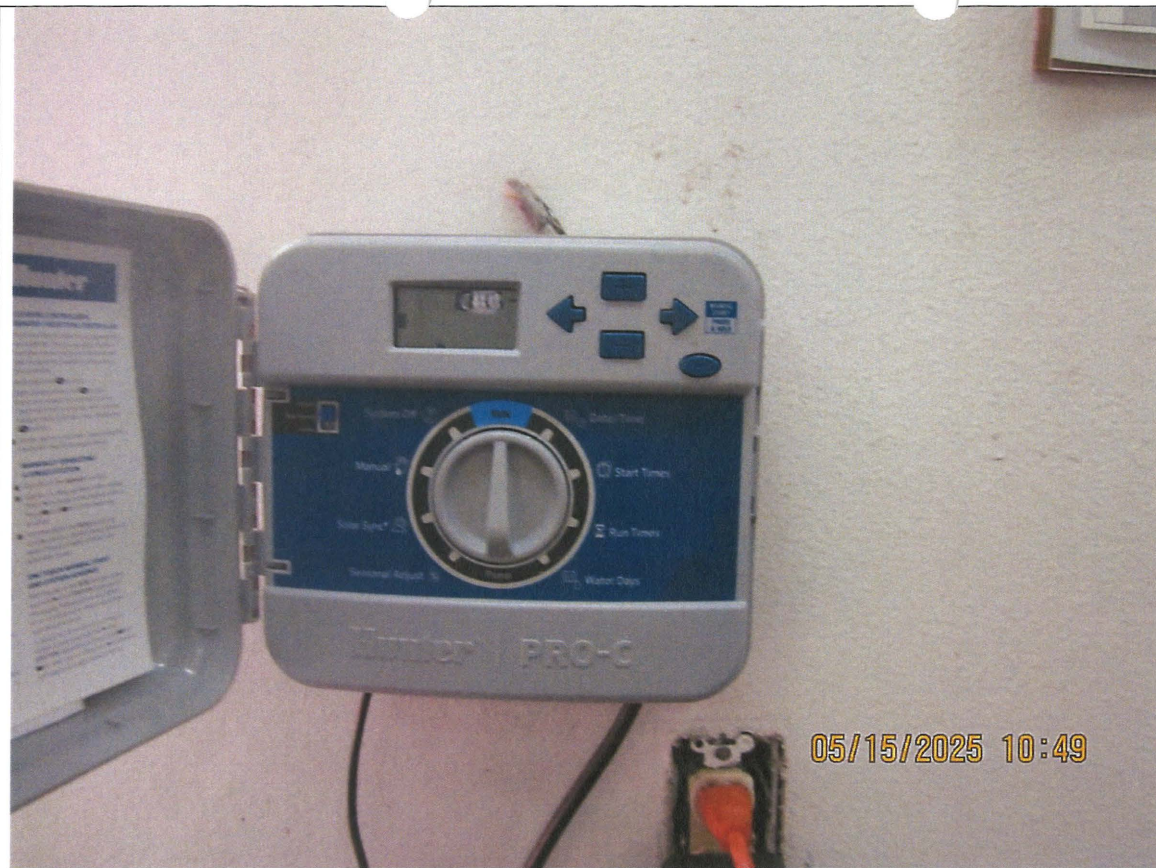
Figure 3. Hunter Pro-C sprinkler control box.
