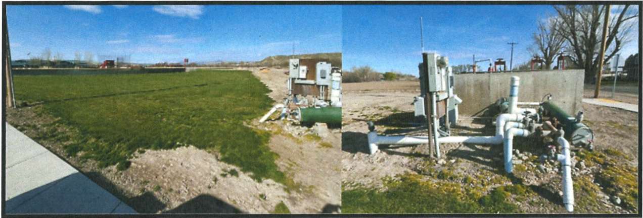
Photos 20 & 21- Surface water pumping station in the northeast corner of the parcel. Providing irrigation to all areas surrounding the baseball fields.
