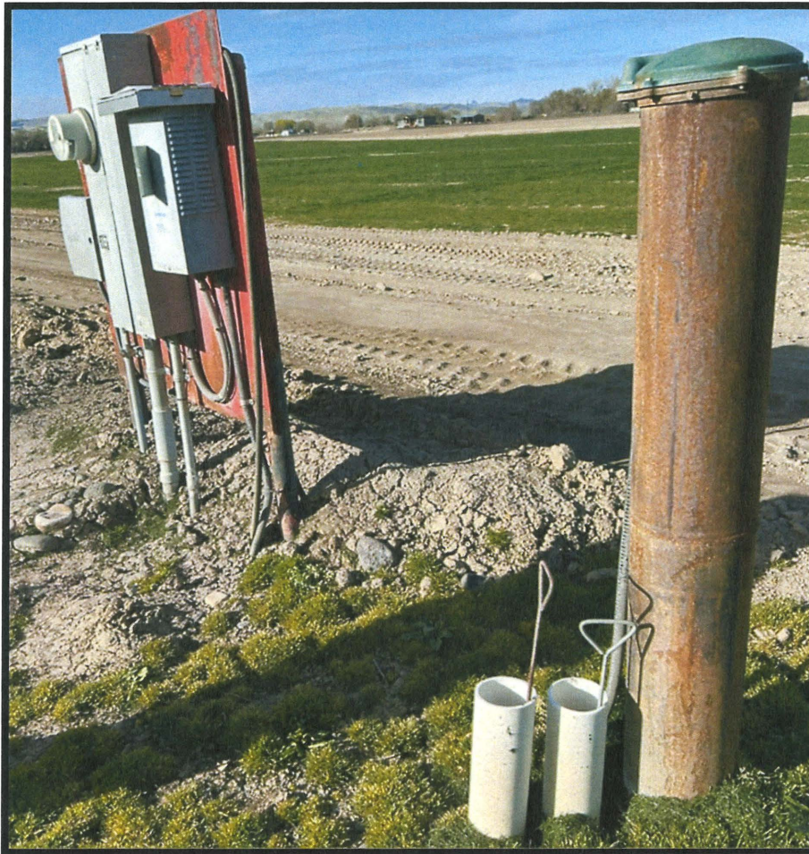
Photo 1- The VFD and power supply on the left of the well head. The drain valve is in the white pipe closest to the casing and the main shutoff valve is in the white pipe on the left of the drain in the image.
