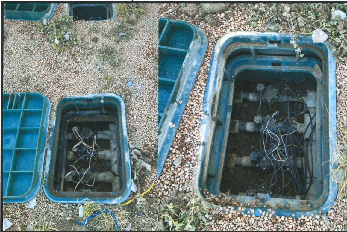
Photos 7 & 8- The control valve boxes for field #1, with 4 valves in each.
