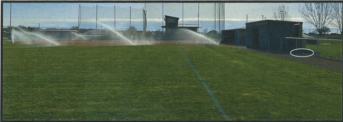
Photo 6- Field #1- the control valve boxes for the field are on the other side of the fence line (circled blue). The irrigation timers for both fields are in the “clubhouse” adjacent to the valve boxes.
