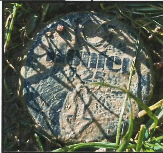
Photo 19- Hunter T-25 sprinkler heads found throughout the baseball fields.
