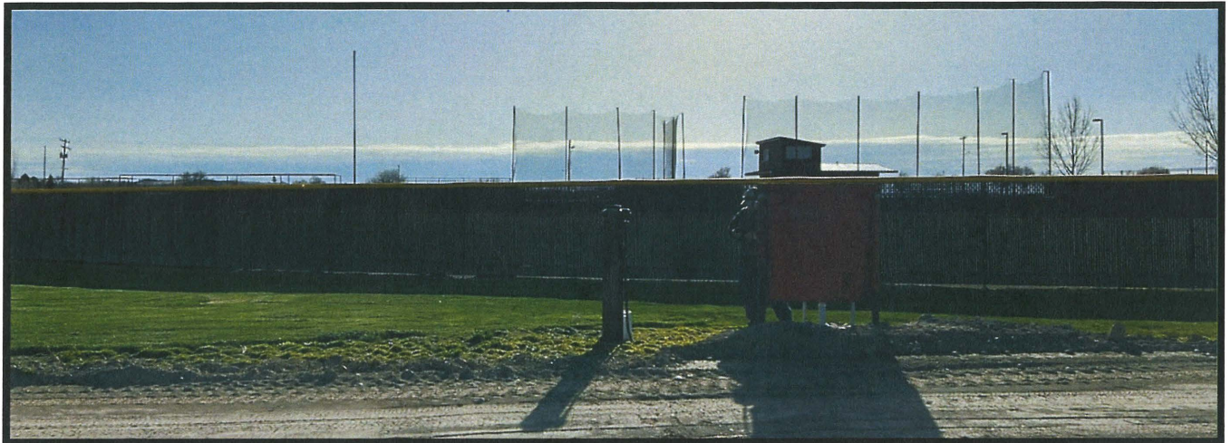
Photo 3- The well head VFD and power supply facing east, both fields' backstops are in the background.
