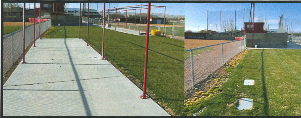
Photos 13 & 14- The control valve boxes for field #2, with 4 valves in each.
