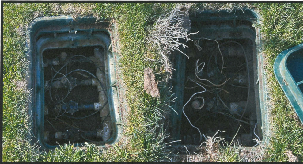
Photo 15- The valve boxes for field #2 with 4 valves in each.
