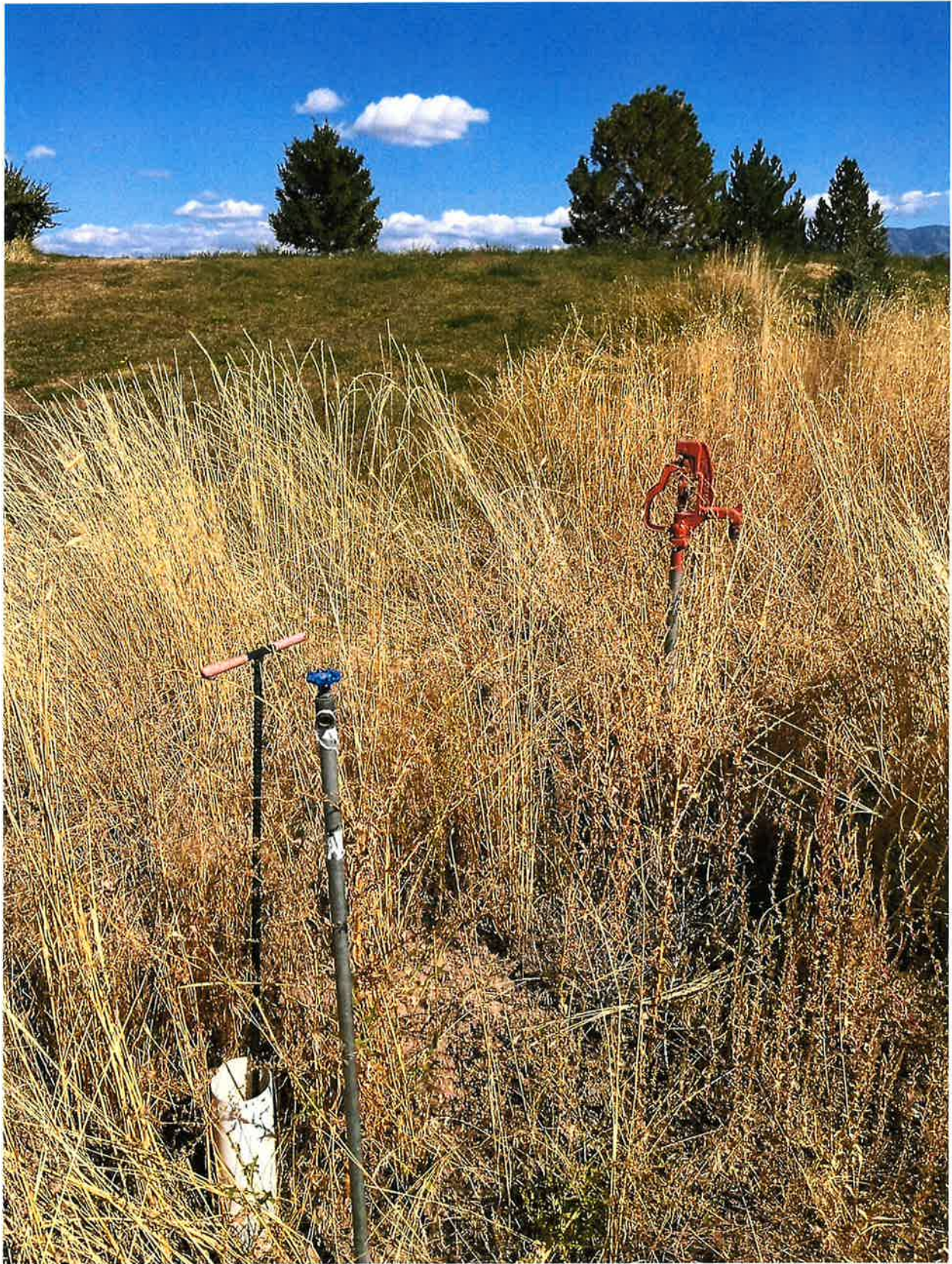
Figure 6 Spigot and frost-free hydrant looking east
