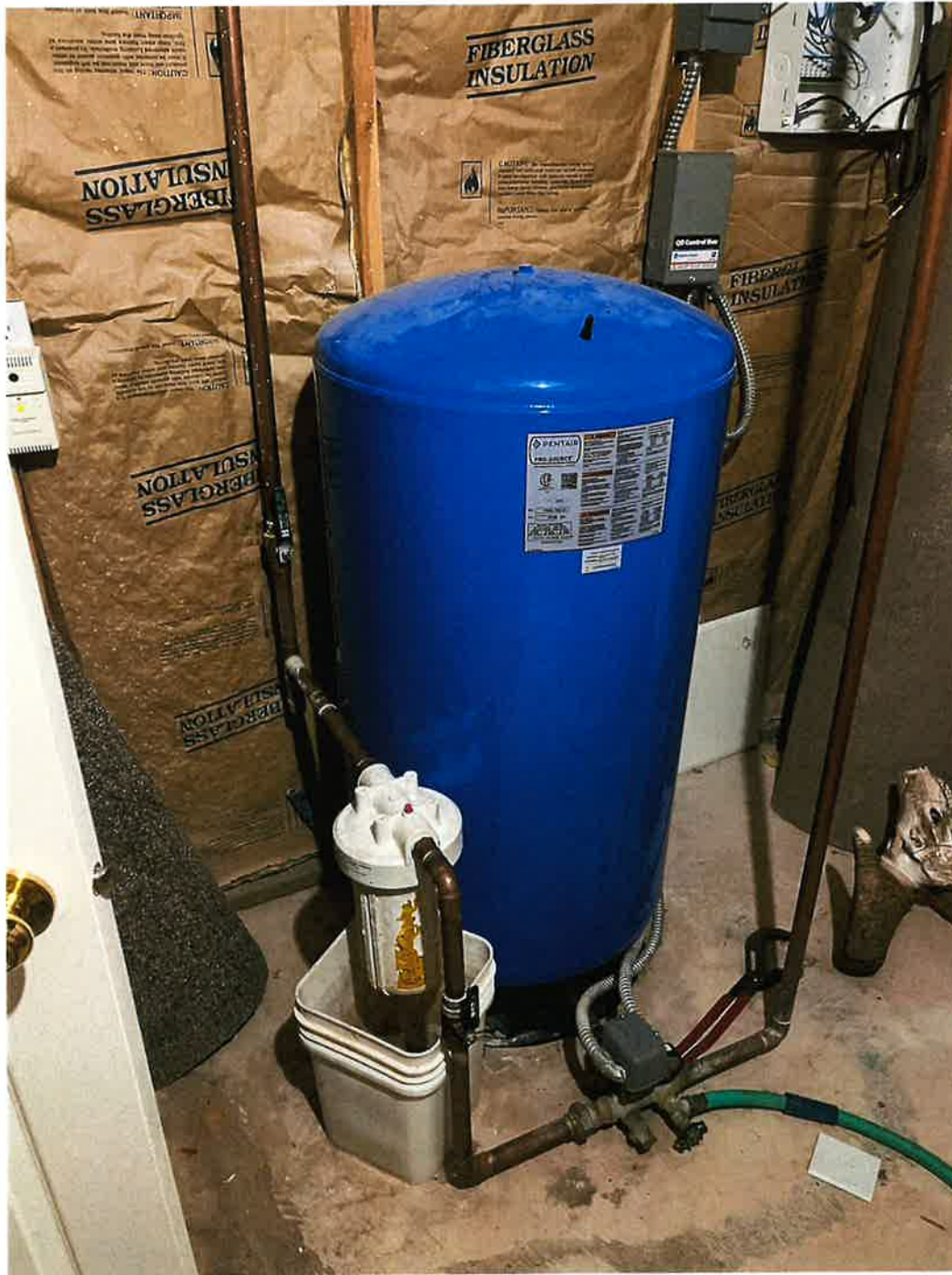
Figure 1 Point of connection in home.
