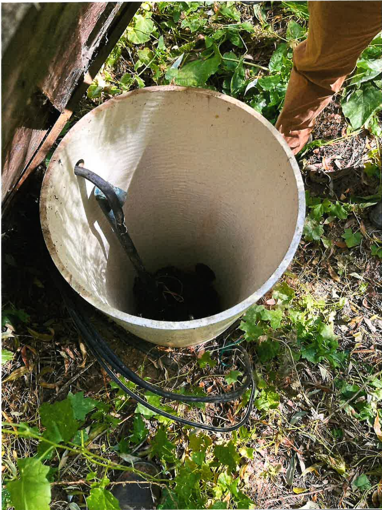
Figure 4 Vertical pipe and pump
