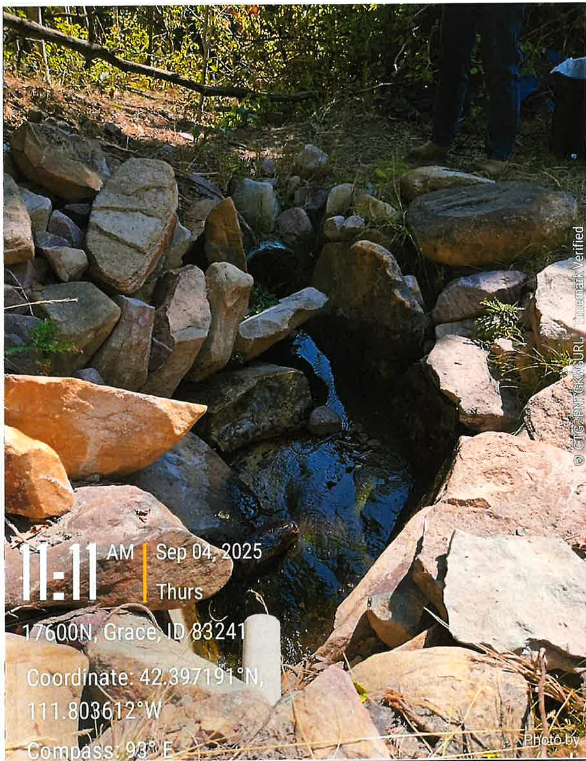
Figure 2 Water flowing into larger pipe
