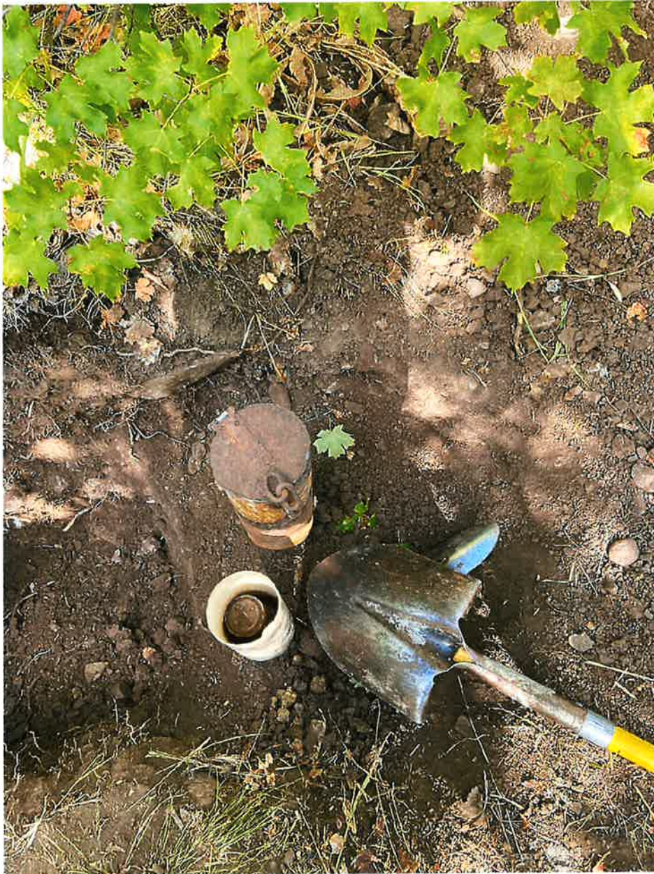
Shutoff valve at the point of diversion for the spring
