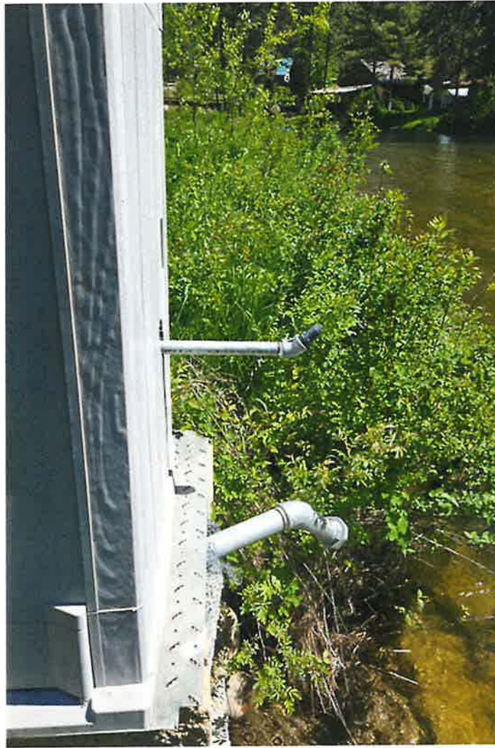
Figure 5 Point of diversion (bottom pipe) and return to public water source (top pipe)
