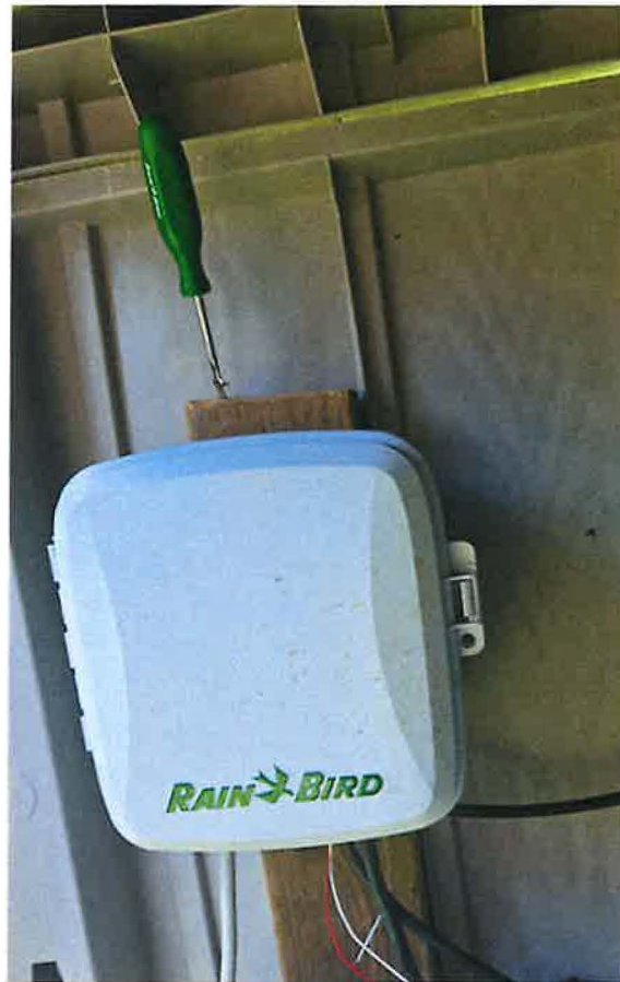
Figure 1 Lockable Rain Bird control panel
