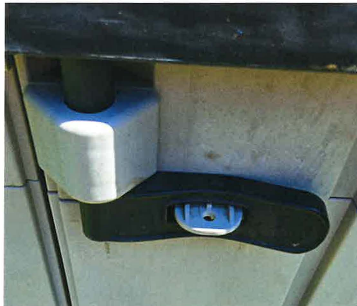
Figure 2 Lockable shed for control panel for pump
