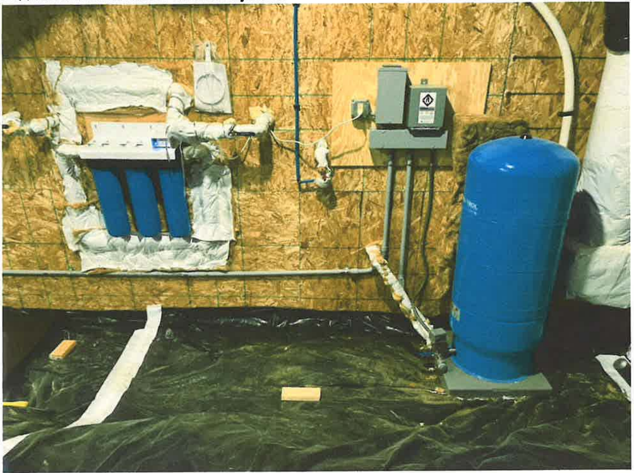
Pressure tank and water filtration system
