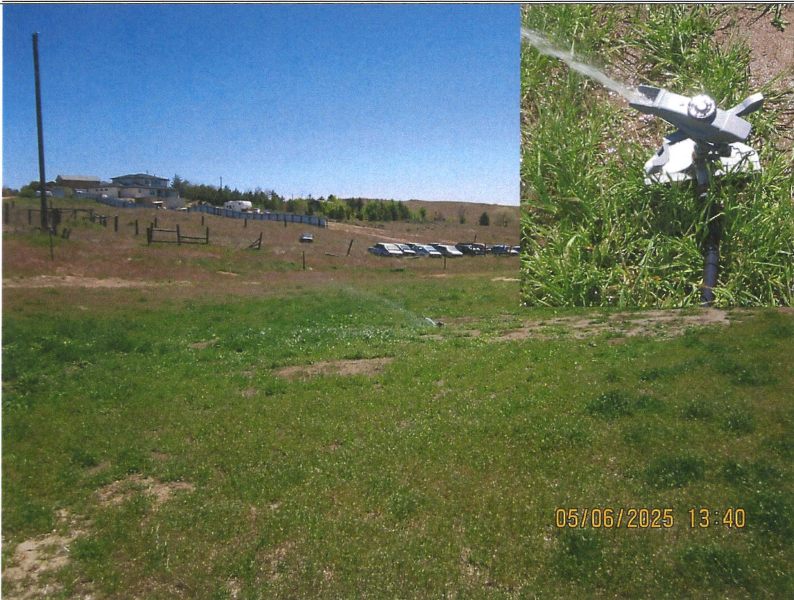
Figure 10. Sprinkler attached to 1-inch black plastic pipe running in pasture.
