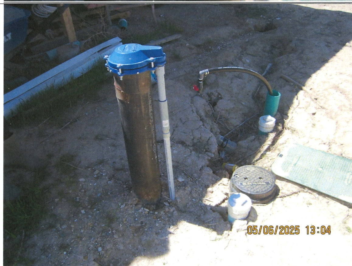
Figure 2. Well head with 6-inch casing
